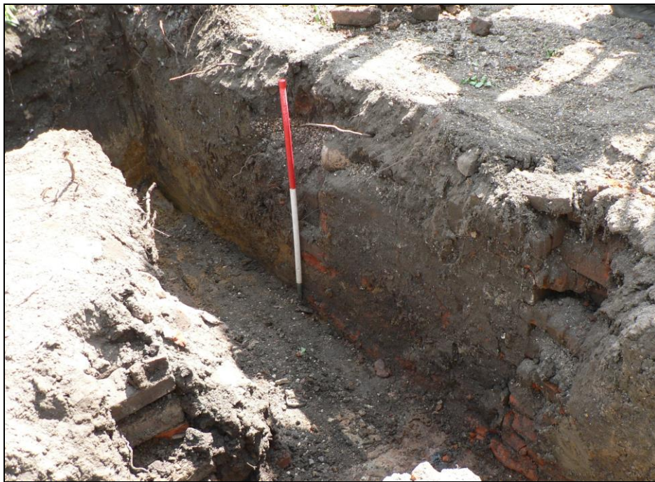
Red brick 19 th century probable small cellar foundation close to south-eastern corner of trenches
