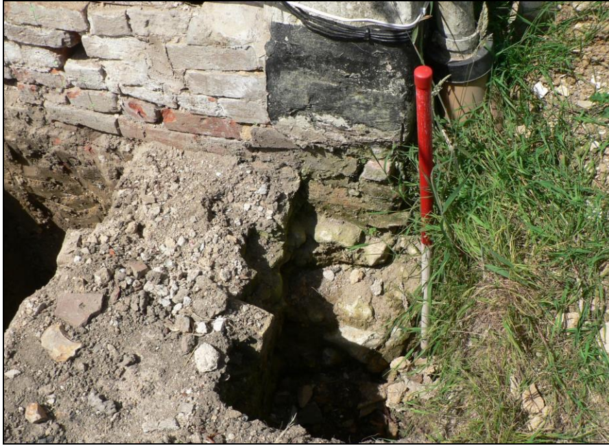
Small section of flint and mortar foundation below north-east corner of building
