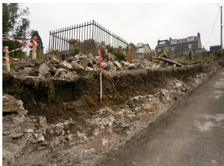
Figure 4c - general image after partial demolition of the wall, leaving the existing foundations
