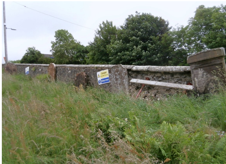
Figure 4a – image showing the partial collapse of the wall prior to dismantling works
