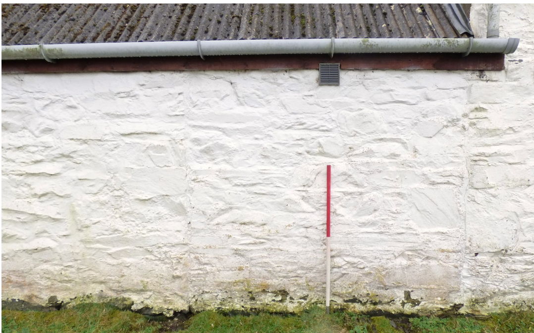
Figure 6c – infilled opening (I) in NW elevation of single storey building (from NW)
