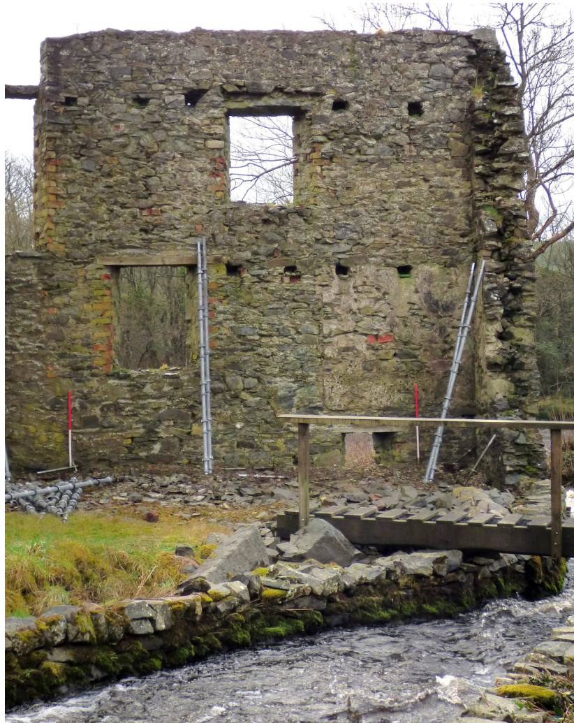
Figure 13a – general of internal SE elevation of 2-storey ruinous building (from NW)
