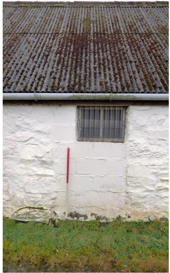
Figure 7b – partially blocked-in opening (II) in NW elevation of single storey (from NW)
