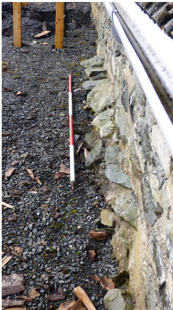
Figure 9b – showing stone protrusions in SE elevation of single storey building (from NE)
