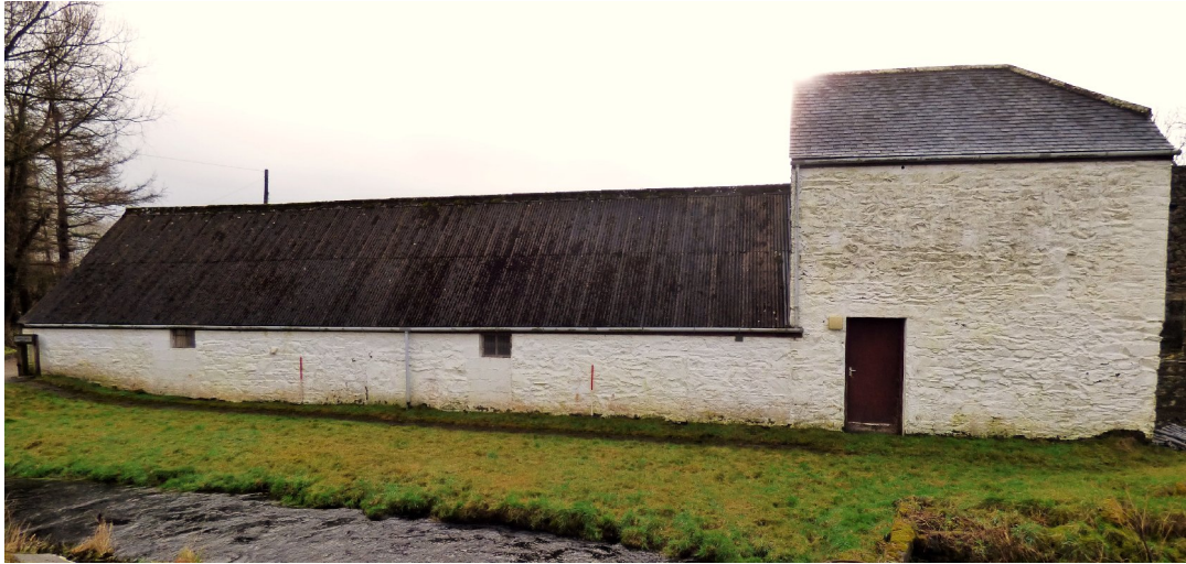
Figure 6a – general of NW elevation of single storey & 2-storey buildings (from WNW)
