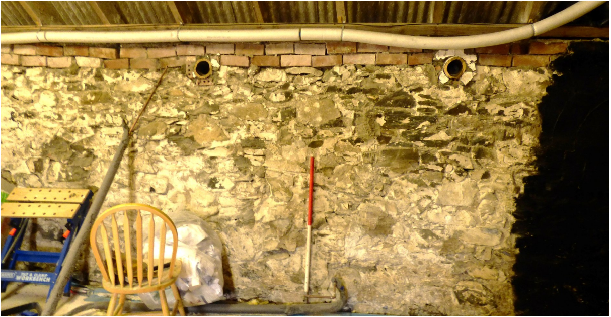
Figure 12a – single storey building (later byre) showing ventilation holes and later brickwork on top of existing stone walls to heighten roof (from NW)
