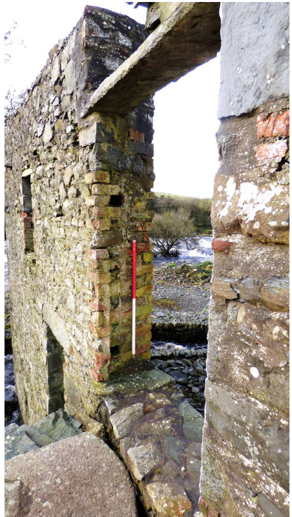
Figure 15c – location of hinges? in entrance of upper storey of ruinous building (from E)
