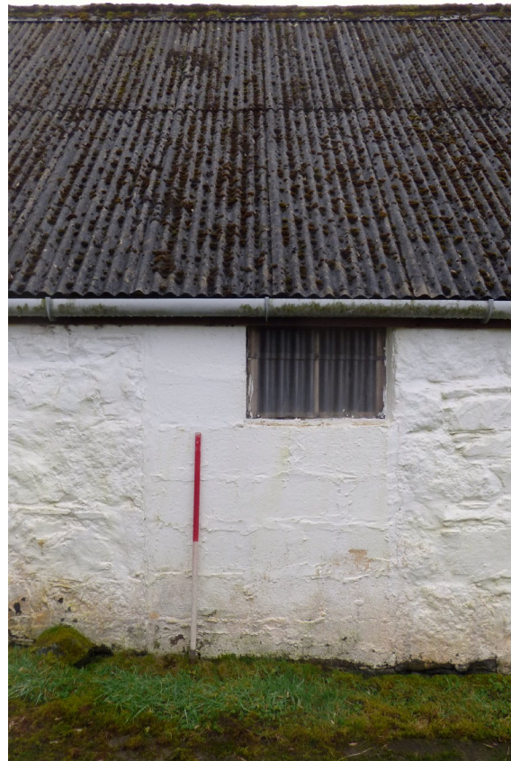
Figure 7d – partially blocked-in opening (IV) in NW elevation of single storey (from NW)
