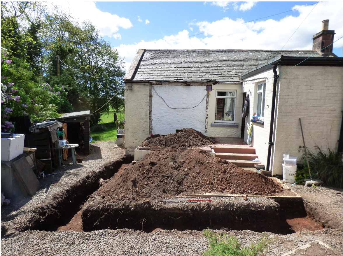
Figure 6b – general pre-ex of proposed extension area after partial ground reduction (from N)
