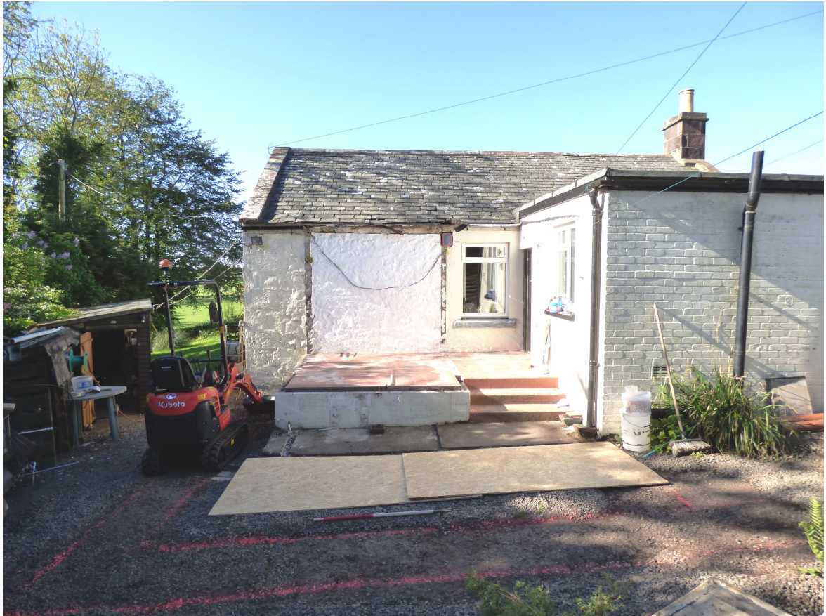
Figure 6a – general pre-ex of proposed extension area after partial ground reduction (from N)
