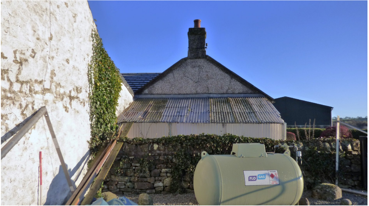
Figure 16a – SW gable & 'greenhouse' structure at SW end - south-eastern range (from SW)
