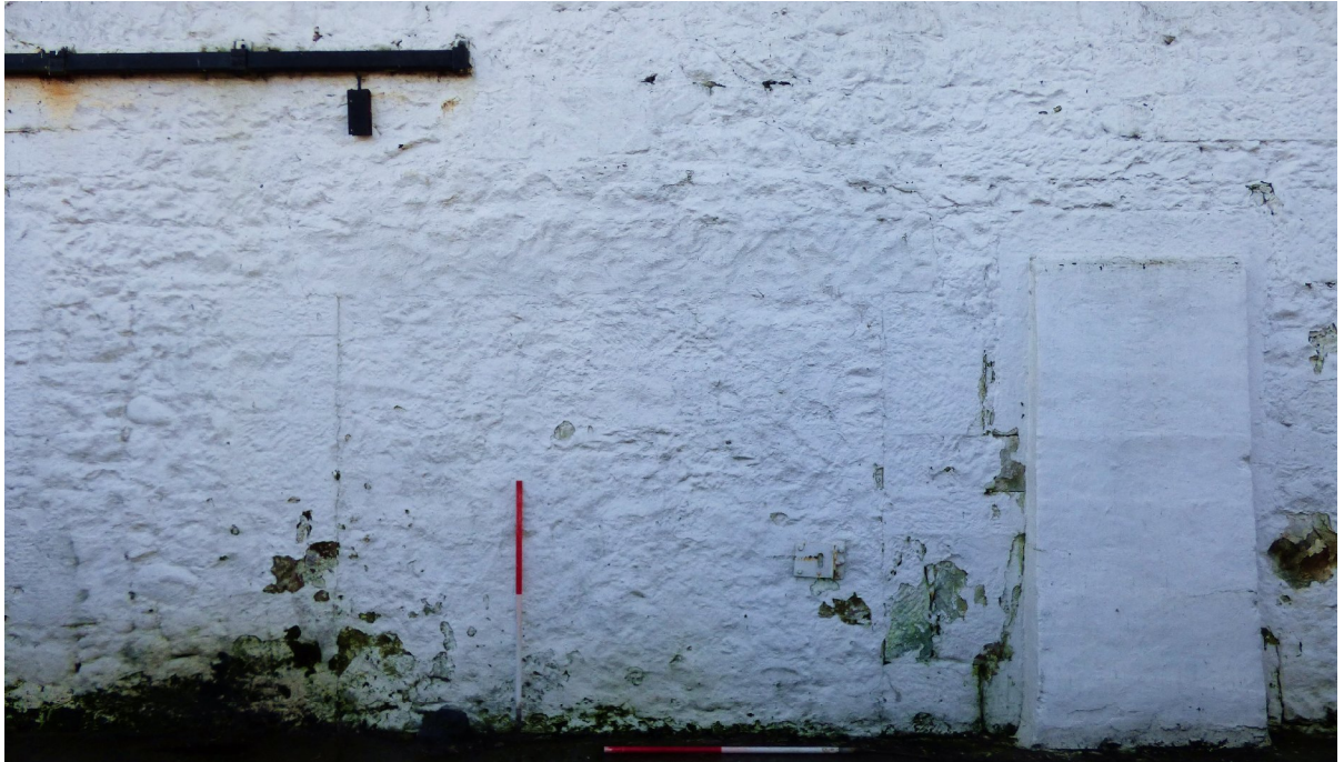
Figure 13a – infilled (large) opening & buttress (in front of former doorway) of NE elevation - south-western range (from NE)
