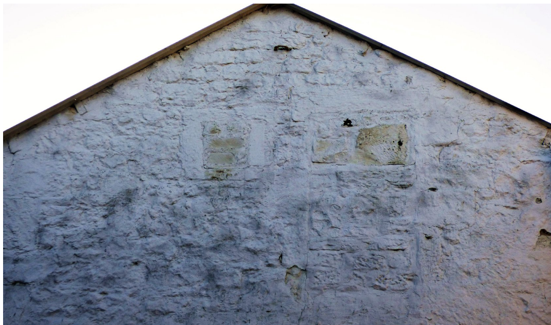
Figure 12b – detail of infilled window & doorway in NW gable - SW range (from NW)
