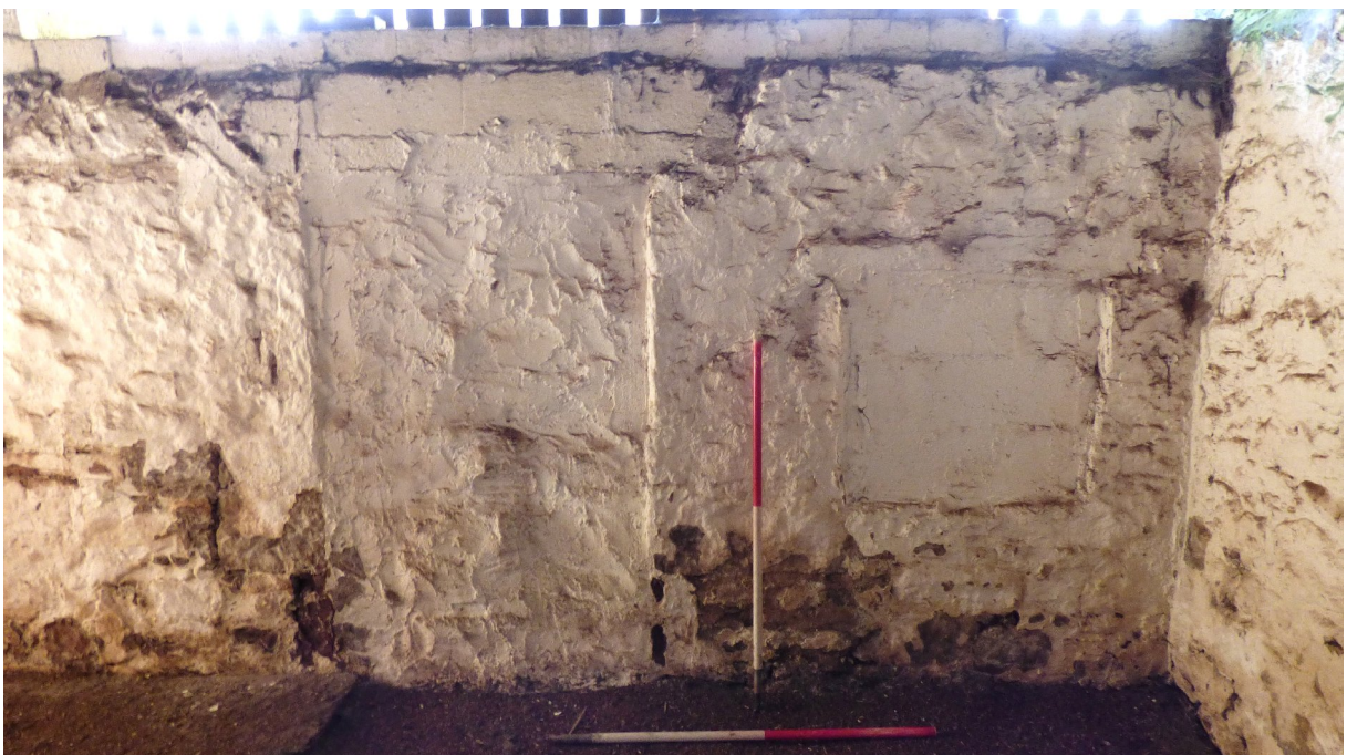
Figure 9c – interior of blocked-in doorway & window in SW elevation - NE range (from NE)
