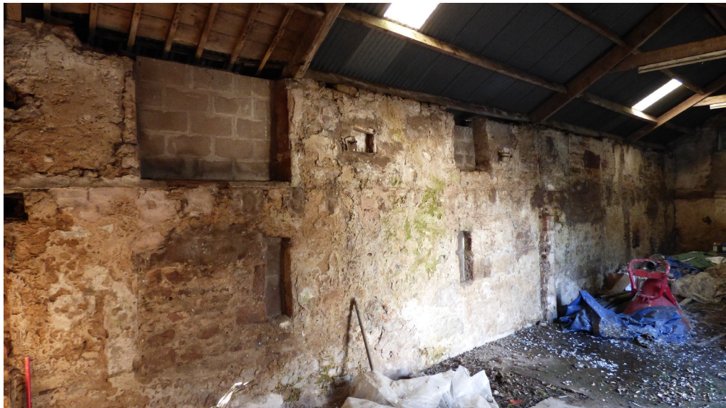
Figure 14b – detail of infilled openings in SW elevation – SW range (from ESE)
