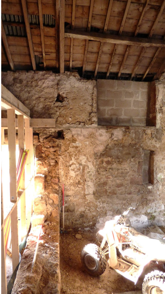
Figure 15a – partially demolished wall at NE end of interior – SE range (from NE)
