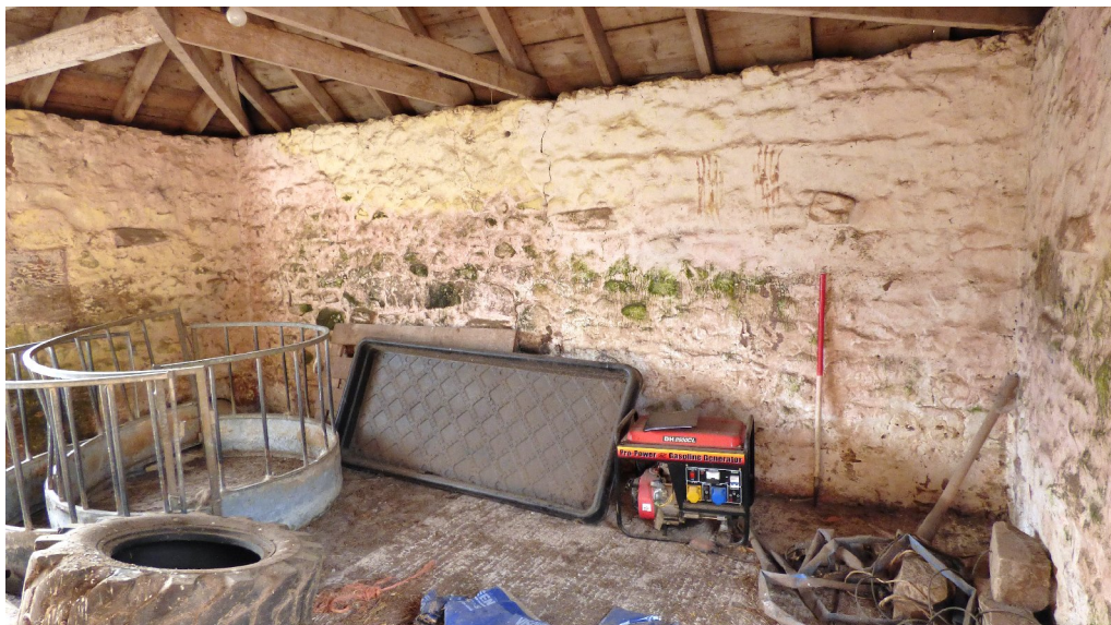
Figure 7b – showing stone protrusions in SW (end) wall - north-western range (from NNE)
