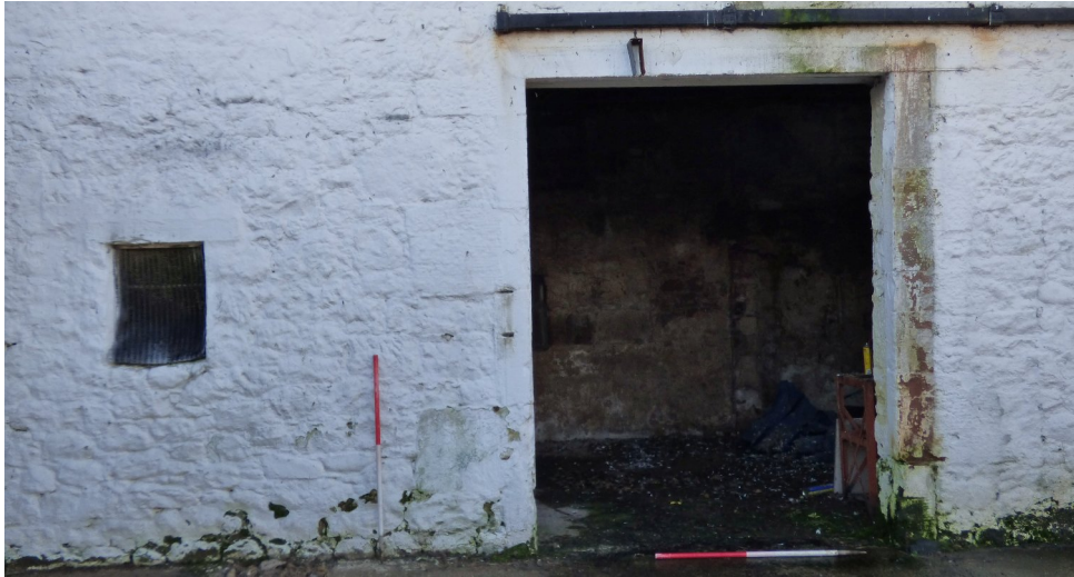
Figure 12a – vent / former window (II) at SE end of NE elevation - SW range (from NE)
