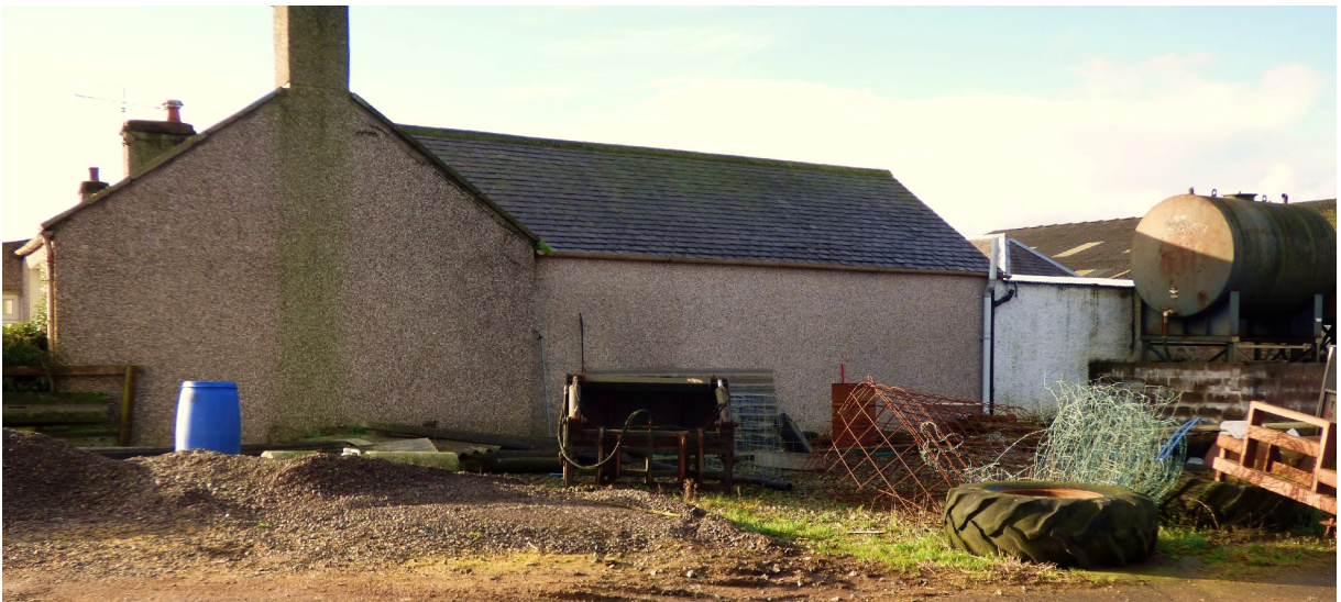
Figure 17b – NE elevation - north-eastern range (dwelling & part of car port) (from ESE)
