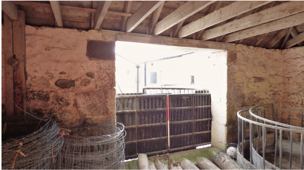
Figure 7a – large entrance at SW end of SE elevation - north-western range (from N)
