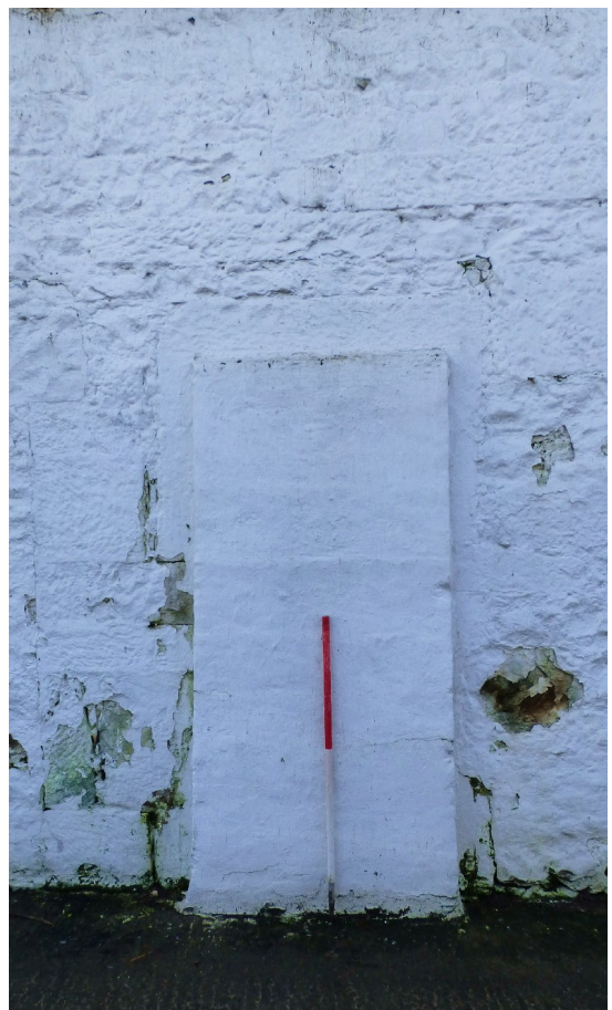
Figure 13c – buttress in front of former doo in NE elevation - SW range (from NE)
