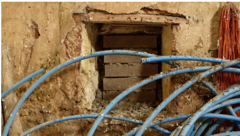
Figure 12c – internal view of blocked-in vent / former window (I) at NW end of NE elevation - south-western range (from SW)
