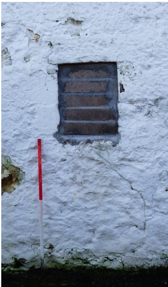
Figure 13b – vent / former window at NW end in NE elevation - SW range (from NE)
