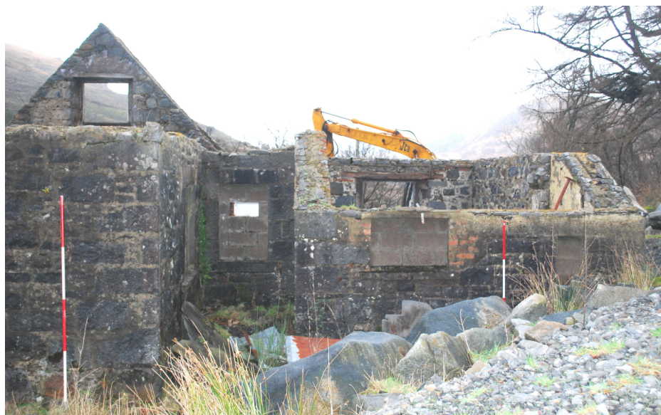
Figure 17c - central area of eastern (rear) elevation showing recessed section between later extension and small extension (from E)
