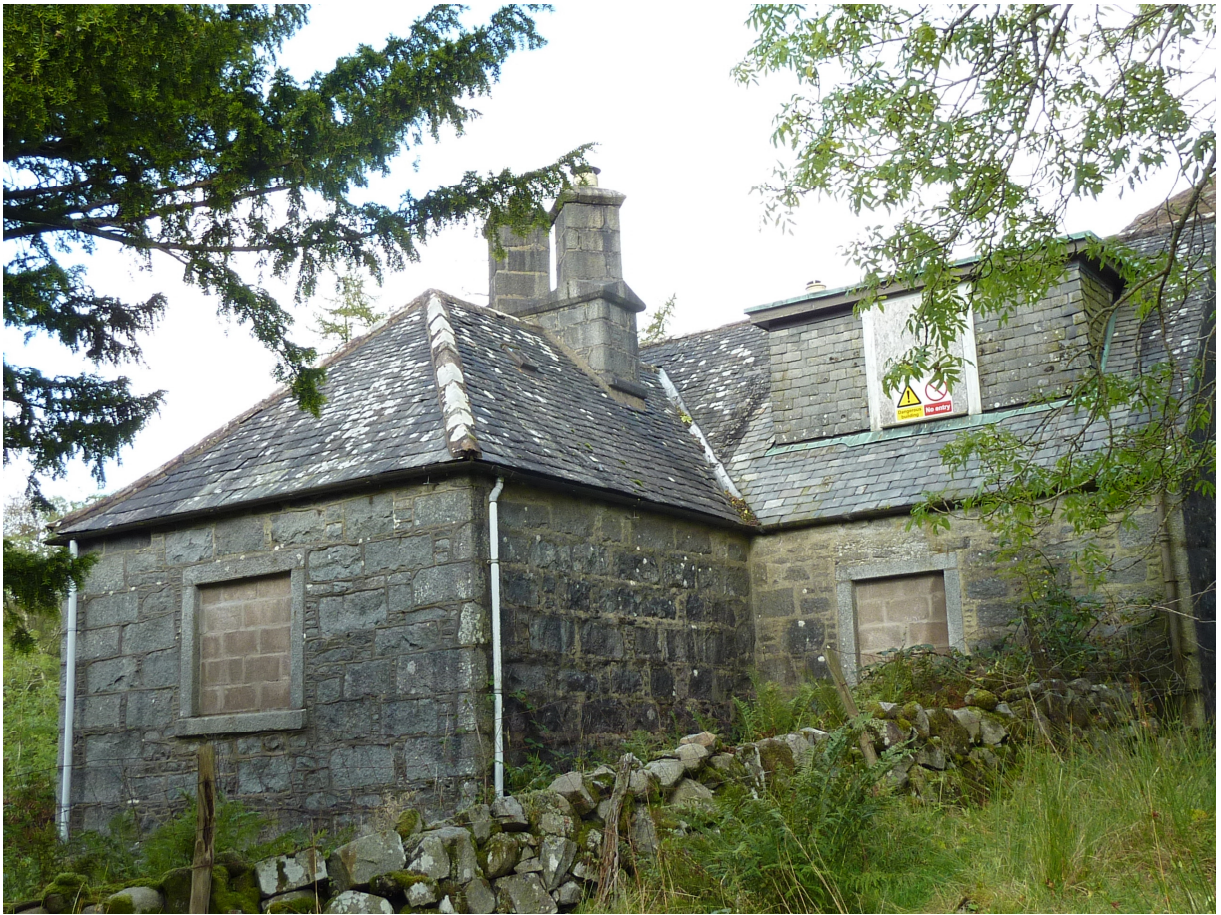
Figure 21a - Glenhead Farm House prior to removal of roof & chimneys (c) Andy Nicholson
