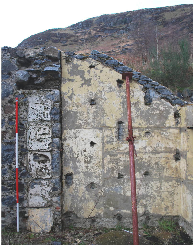
Figure 10b - E-end of northern wall showing where small extension adjoins (from S)
