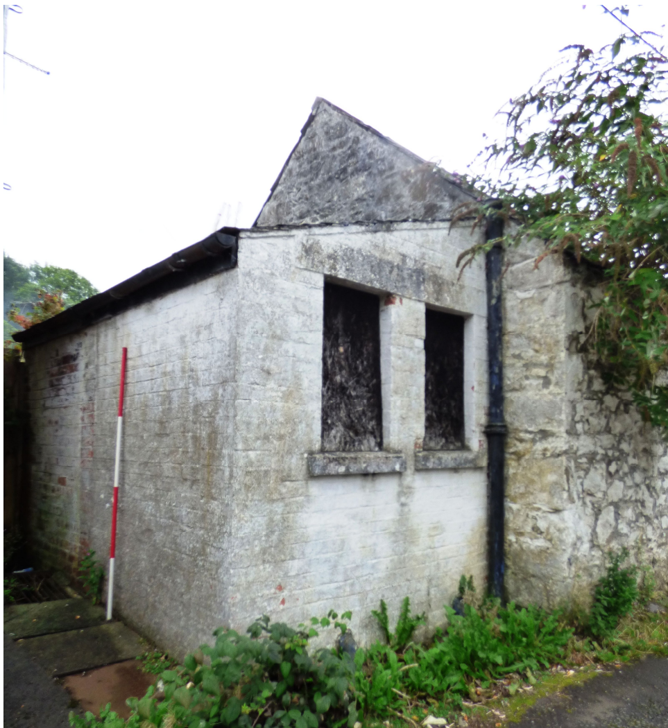
Figure 8c - NNE wall of brick lean-to & part of NNE gable of grain store (from NW)
