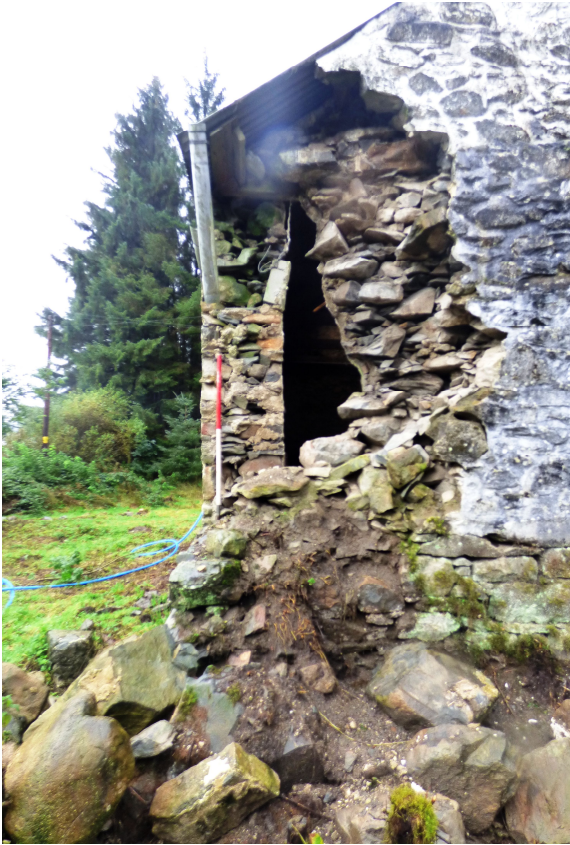
Figure 15a - E corner prior to repair (from NE)
