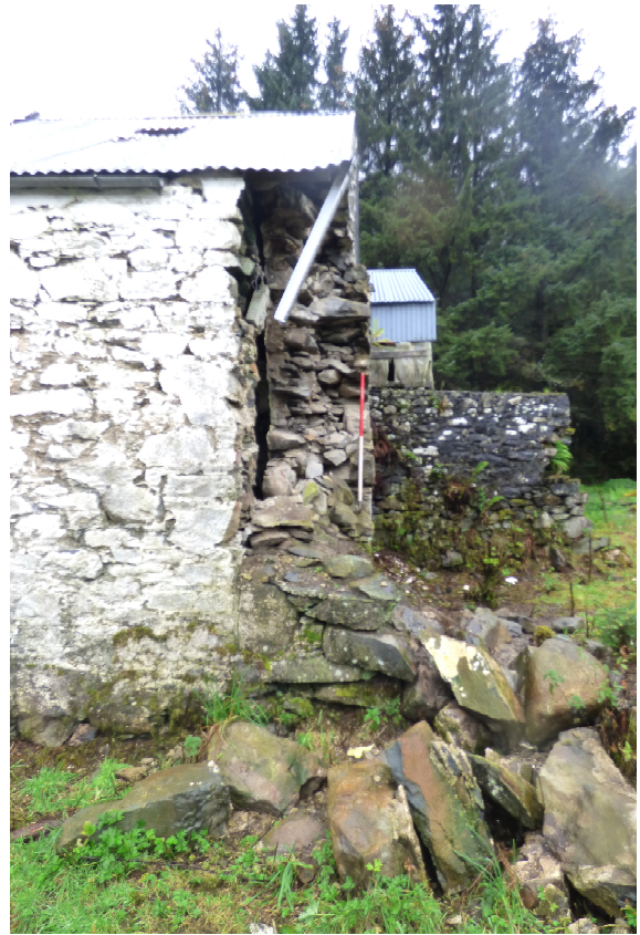
Figure 15b - E corner prior to repair (from SE)
