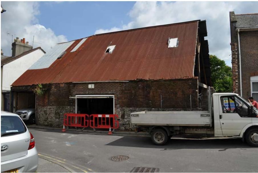
Plate 1: View of site prior to demolition of nineteenth century barn, looking east.
