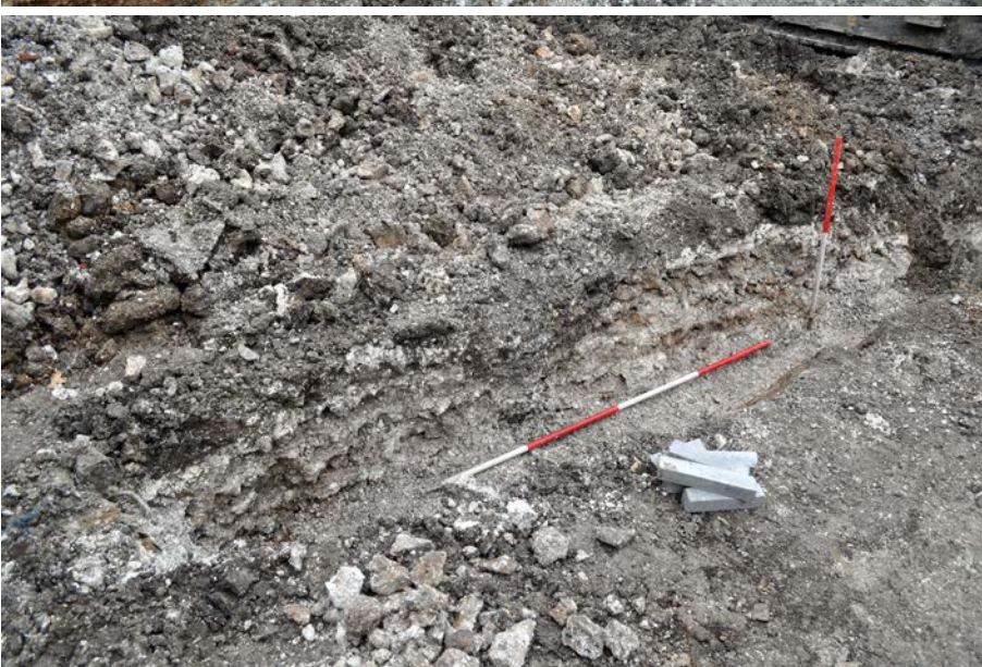
Plate 9: Wall Footing 170 cut through by central footings trench of Trench 5, looking north west. 1m and 2m scales.
