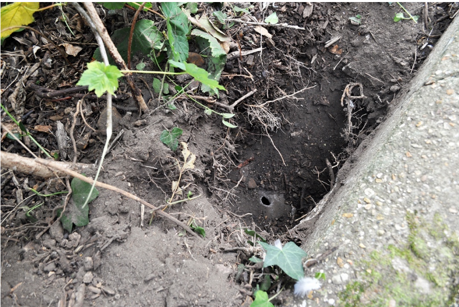
Plate 8: Detail of Hole 124, showing stone slab at base with hole pierced through it by fencing contractors.
