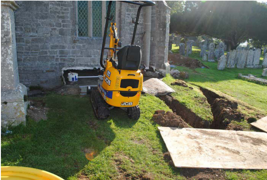
Plate 1: Trenching works adjacent to the West Tower and South Aisle. View from the west.
