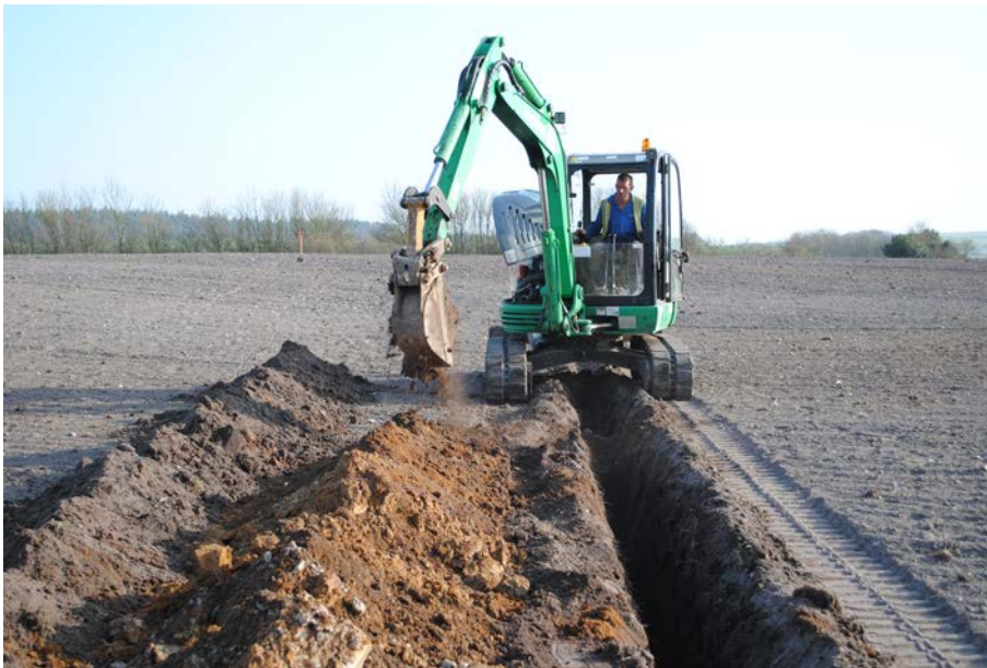
Plate 2: Trenching on rising ground in the south field, viewed from the north.
