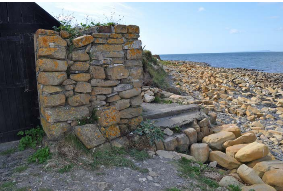
Plate 3: View of stone wall of boathouse and the remains of the former hard wall below to the right.
