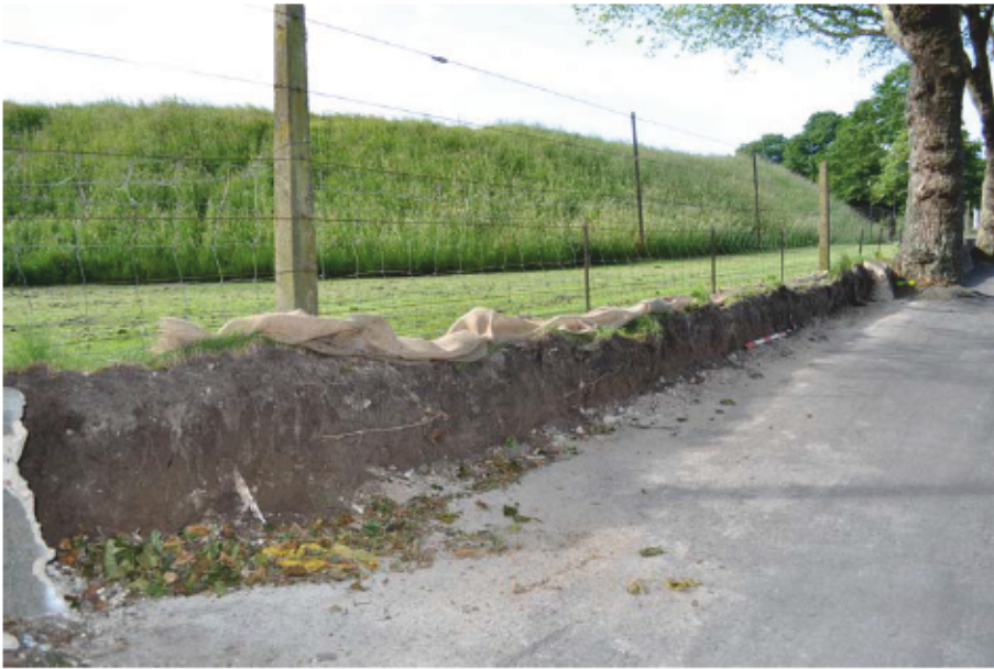
Plate 1: View of soil profile after removal of retaining wall along Weymouth Avenue.
