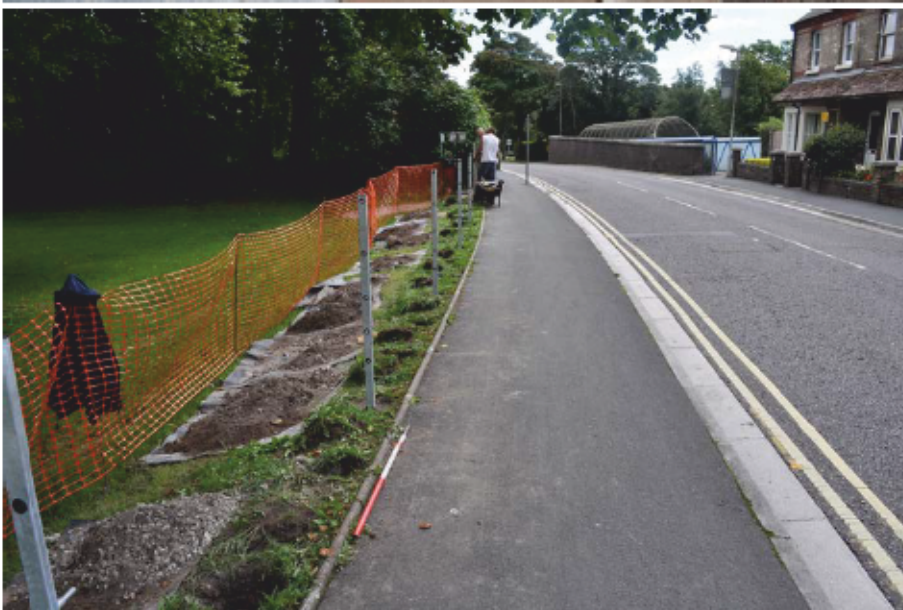
Plate 2: General view of new fence along Maumbury Road, showing postholes and retained spoil behind.
