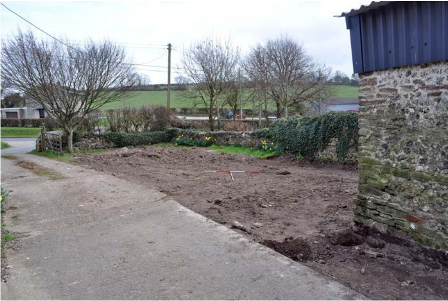
Plate 1: View of new parking area after stripping, looking north east. 2m scales.
