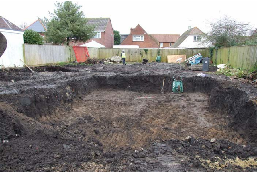
Plate 3: Excavation of basement area in progress, with remnants of layer 107 exposed. 1m scale. View from west.
