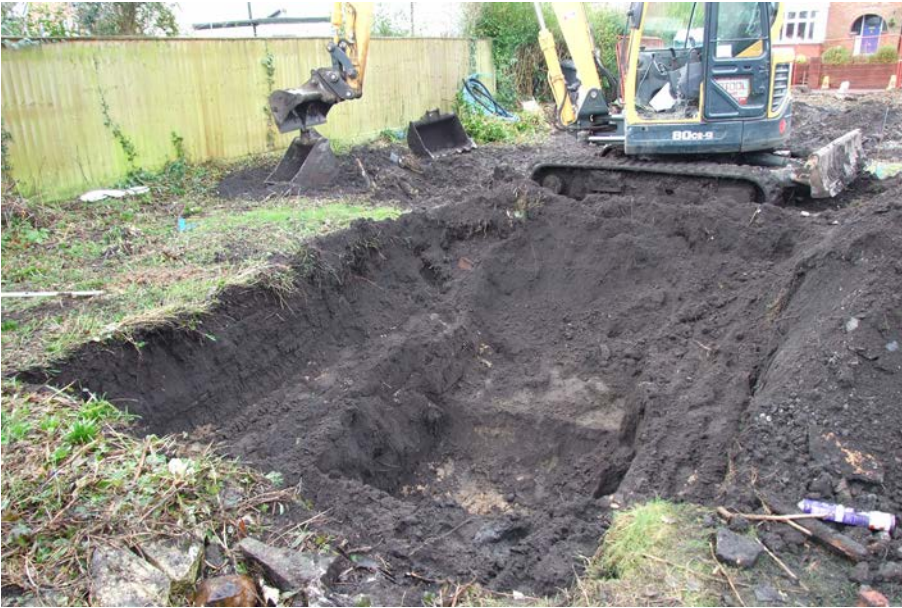
Plate 1: Stepped excavation of soil-percolation test pit at the east end of the site. View from east.
