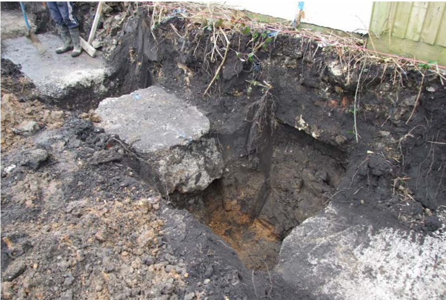
Plate 2: Excavation of segmented footing pits adjacent to neighbouring property to north. View from SSE.
