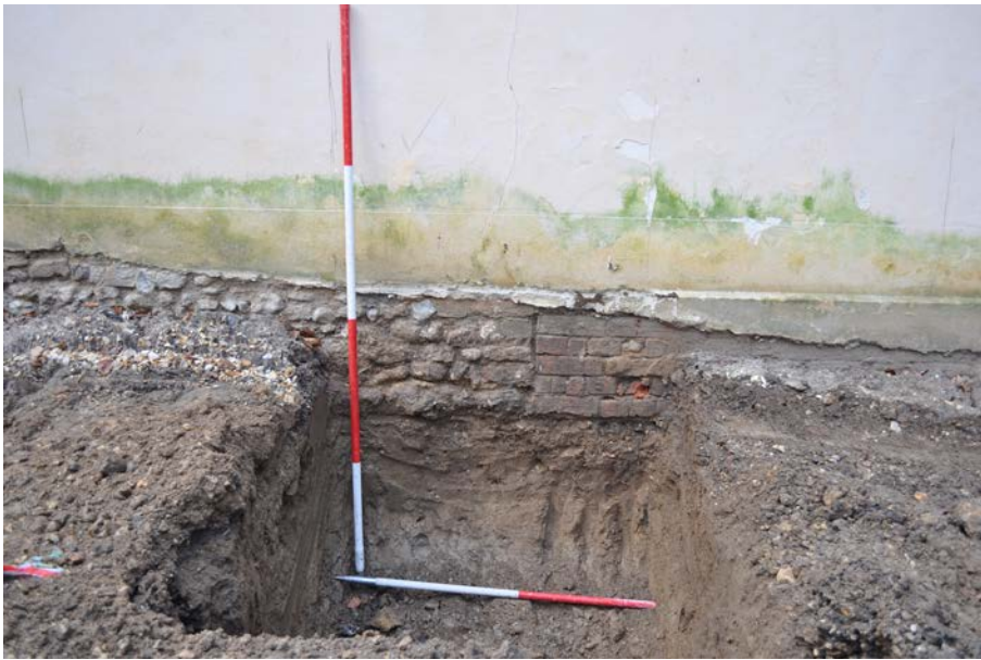
Plate 4: Junction between base of walls in original cottage (right) and later extension (left) in underpinning pit 9. 2m and 1m scale.
