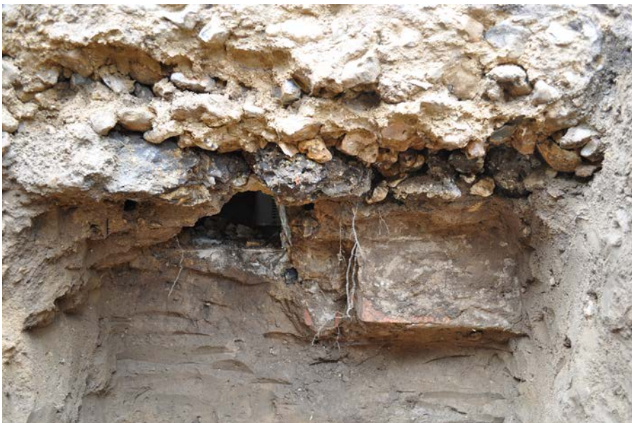
Plate 8: Detail of base of footing 105, with bricks of structure 109 to right and gap formed by removal of slate (111) to left, exposed in underpinning pit 12.
