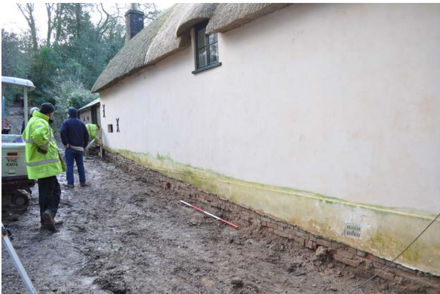
Plate 2: East wall of cottage showing the brick plinth to the north and flint base to the south, below the level of the render, looking SSW. 2m scale.
