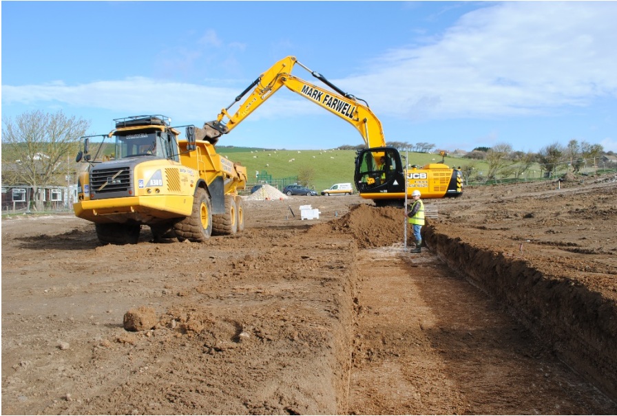
Plate 4: Secondary ground reduction works for the new school building. View from south.
