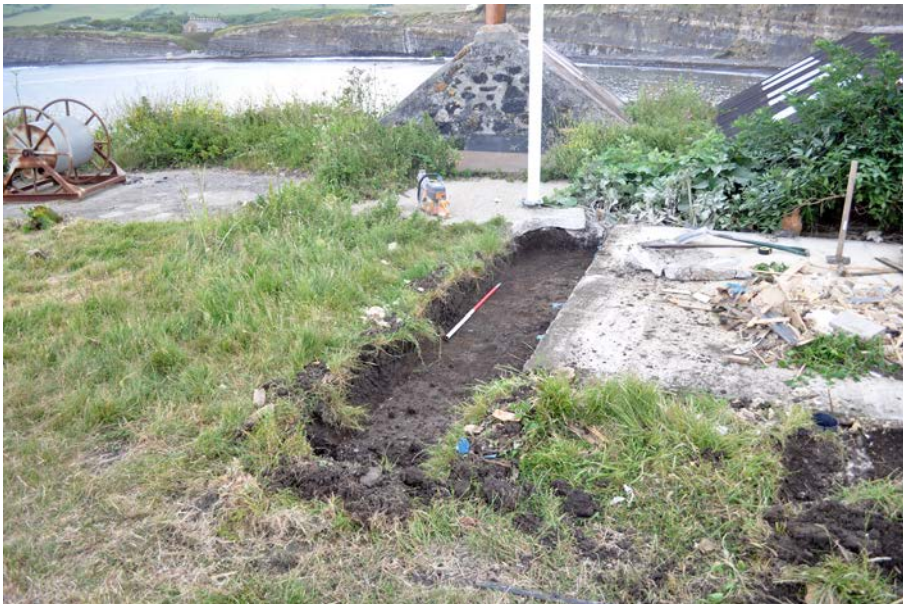
Plate 2: West side of concrete base after excavation, viewed from south. 1m scale.
