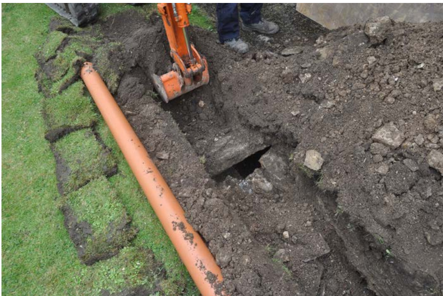
Plate 5: Vault entrance 126, with capstone 125 partially dislodged by machine. View from north west.
