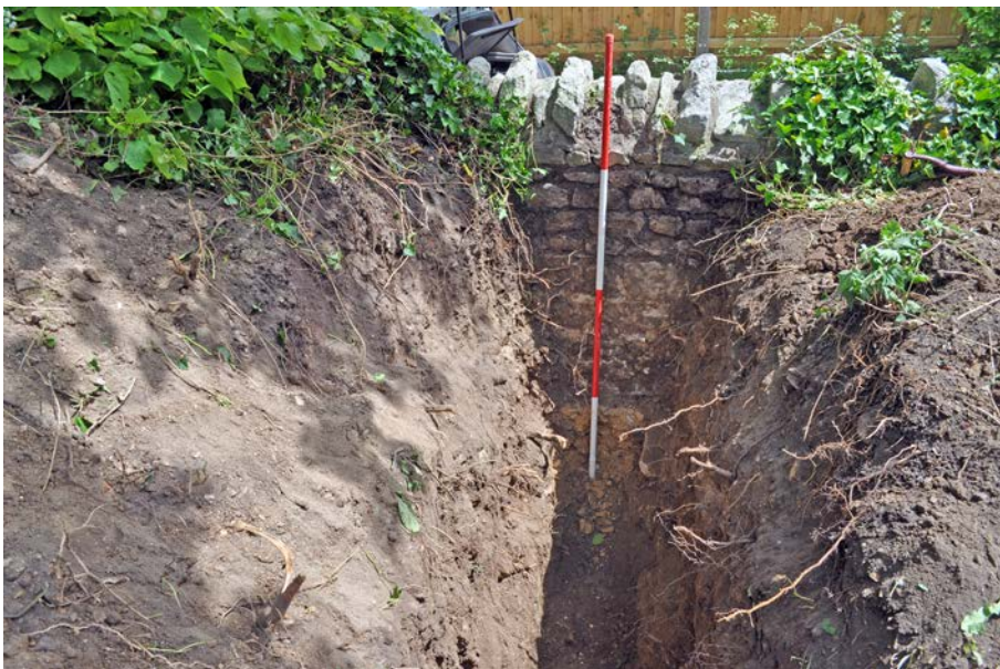
Plate 11: Rear face of churchyard wall and footings 135. 2m scale. View from west.
