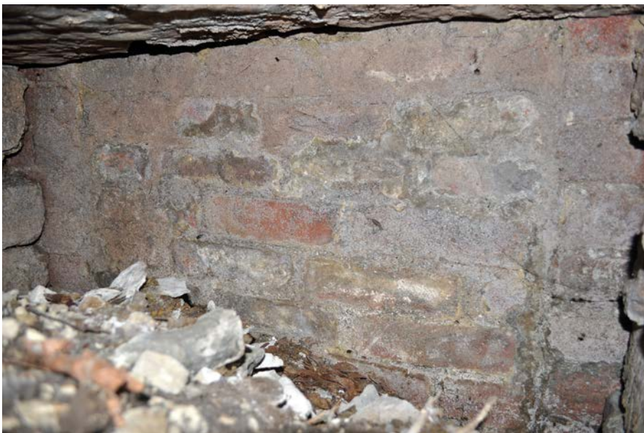
Plate 8: Blocking 127 in north wall of nave, within vault entrance 126. Viewed from north west.
