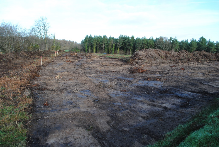
Plate 1: Overview of Lowdens Copse during stripping of PAWS topsoil. View from the south east.
