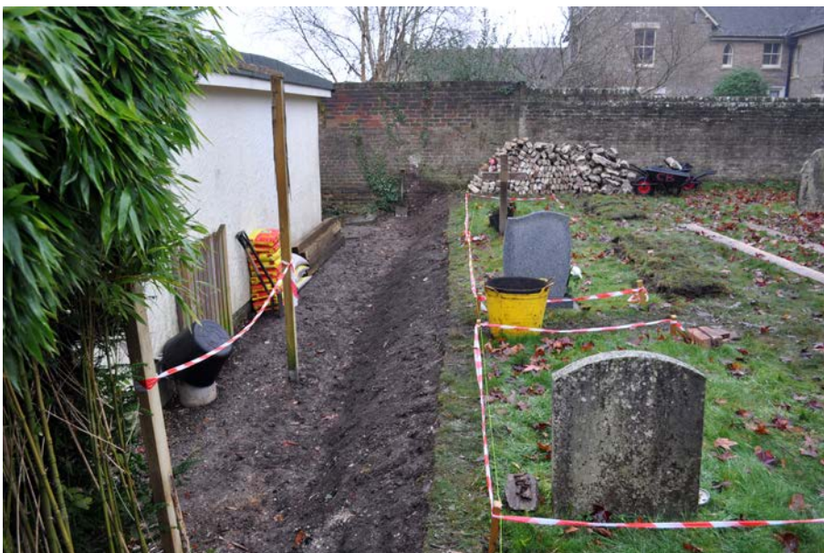
Plate 3: View east along site after battering of churchyard soil, prior to erecting fence.
