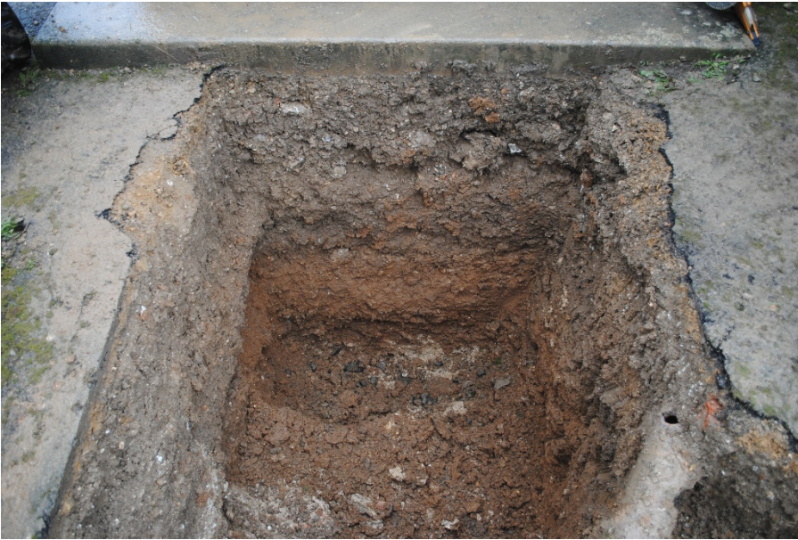
Plate 4: Soil sequence exposed in the south west face of the new soakaway pit. View from north east
