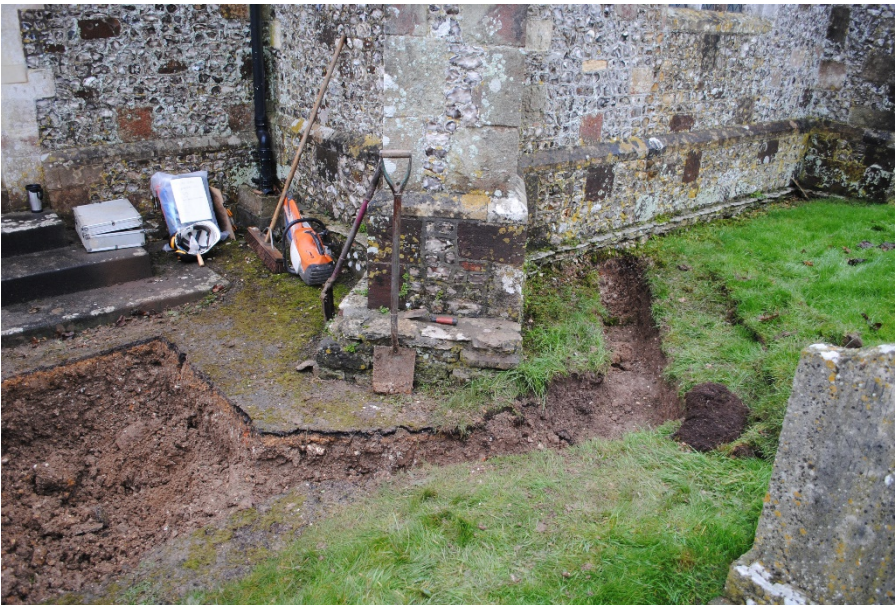
Plate 2: Detail of new service trench linking North Aisle to new soakaway. View from east.
