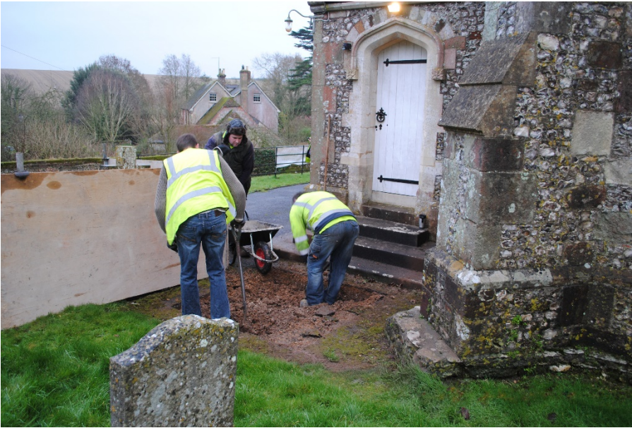
Plate 1: Overview of works showing location of new soakaway pit outside vestry. View from north.
