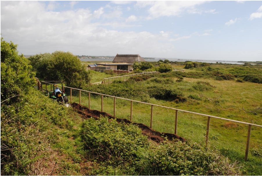
Plate 4: Pipe trenching works immediately east of the Double Dykes. View from west
