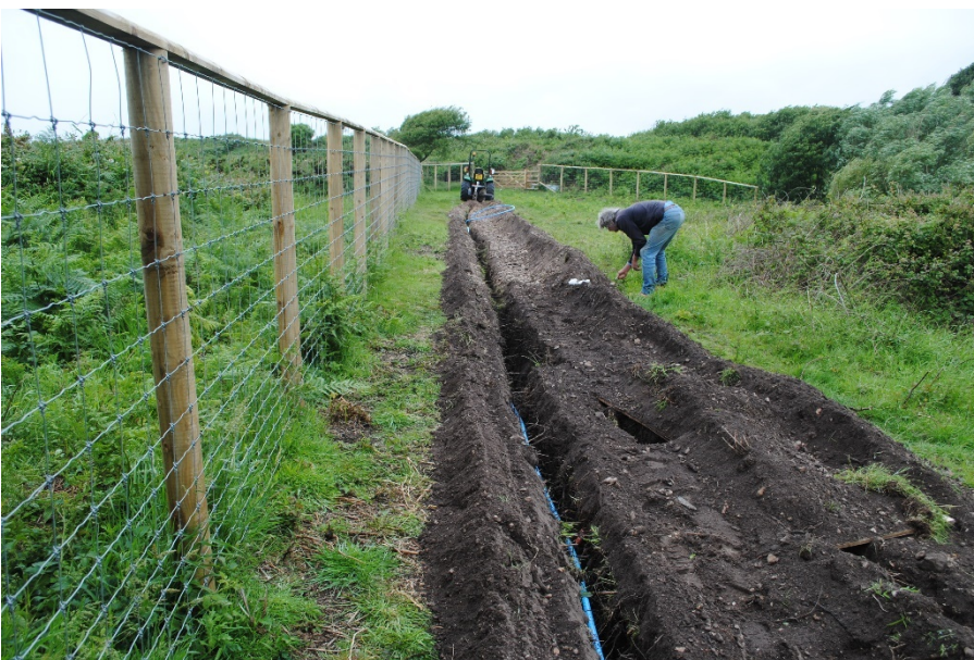
Plate 2: Pipe trench excavation in progress south of the Visitor Centre. View from east.
