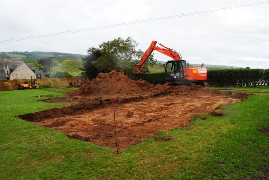
Plate 2: Initial topsoil stripping of the new house footprint area. View from east.
