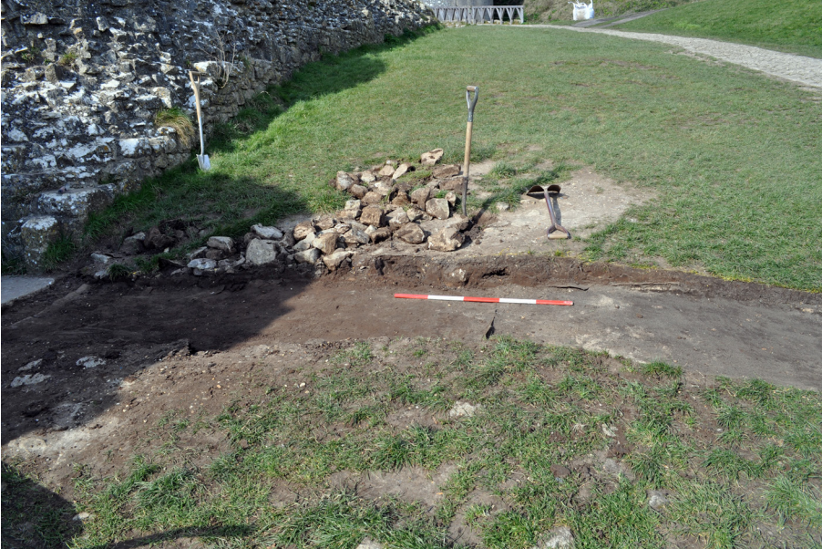
Plate 2: West end of Trench 1 after removal of rubble infill 102 showing geotextile membrane below. Viewed from South. 1m scale.
