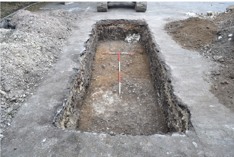
Plate 3: Road gravels etc after initial cleaning. Viewed from West. 1m & 2m scales.
