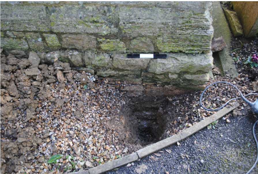
Plate 2: Test Pit 2, showing foundation of the west Nave wall. View from west. 0.3m scale.
