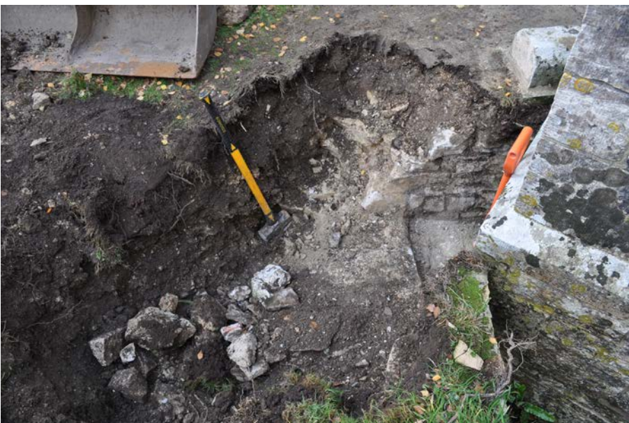
Plate 3: Revetment wall 105 partially destroyed for new drain, looking south.
