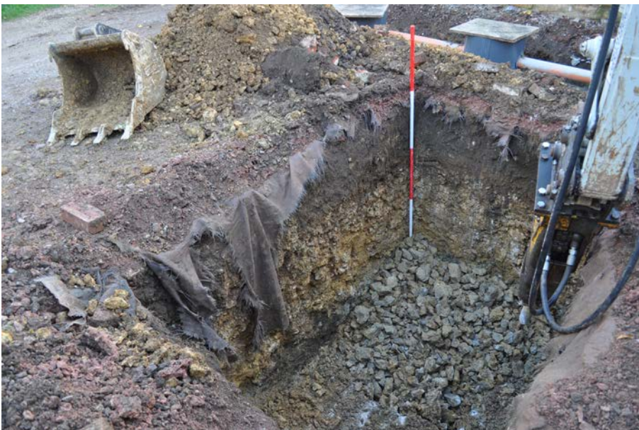
Plate 5: Trench 2 during excavation (breaking up the stone in base of trench), looking south-east. 2m scale.
