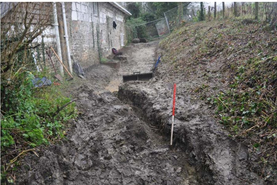
Plate 3: General view of site after excavation of drain trench, looking north. 1m scale.
