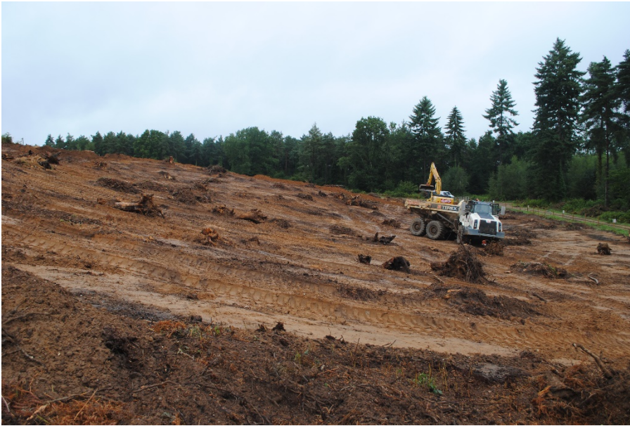
Plate 1: Overview of site during stripping of PAWS soil prior to stump removal. View from the south.
