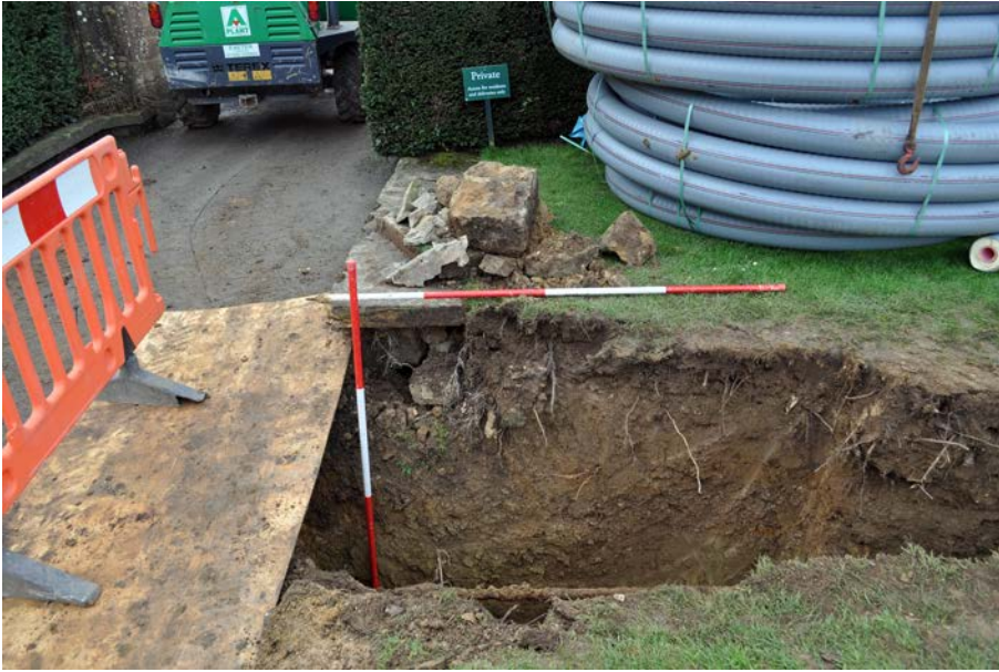
Plate 7: New heat main trench where it cuts through lawn re-vestment wall 115, viewed from ENE. 2m scales.
