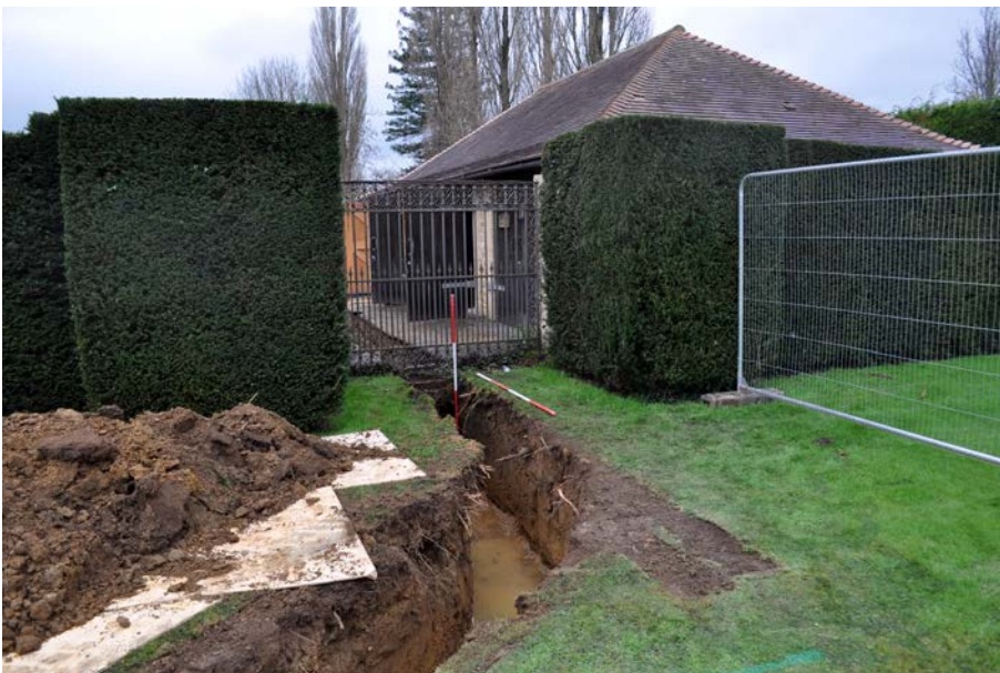
Plate 2: New heat main trench running from garages into north lawn, viewed from ENE. 2m scales.
