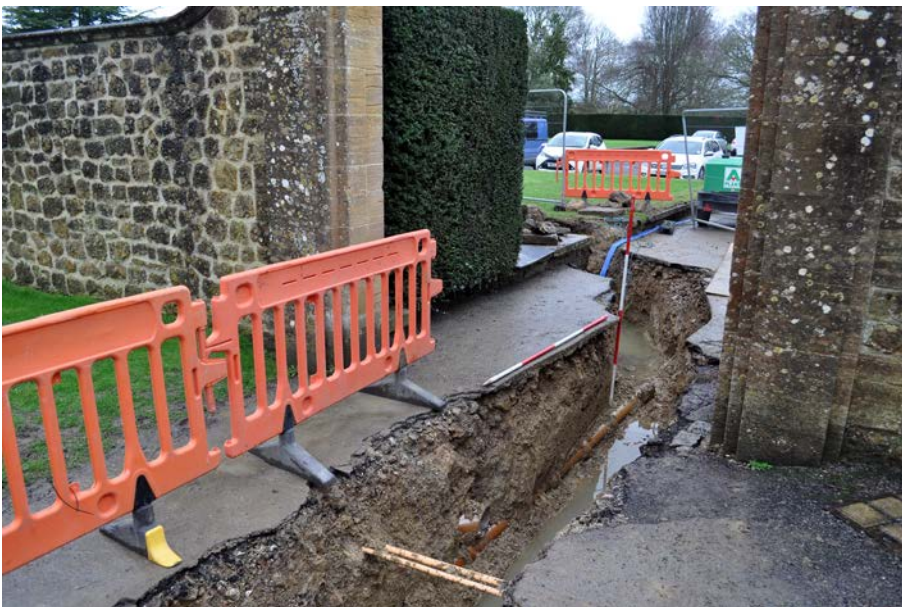
Plate 8: New heat main trench along road, showing drains and services, viewed from SW. 2m scales.
