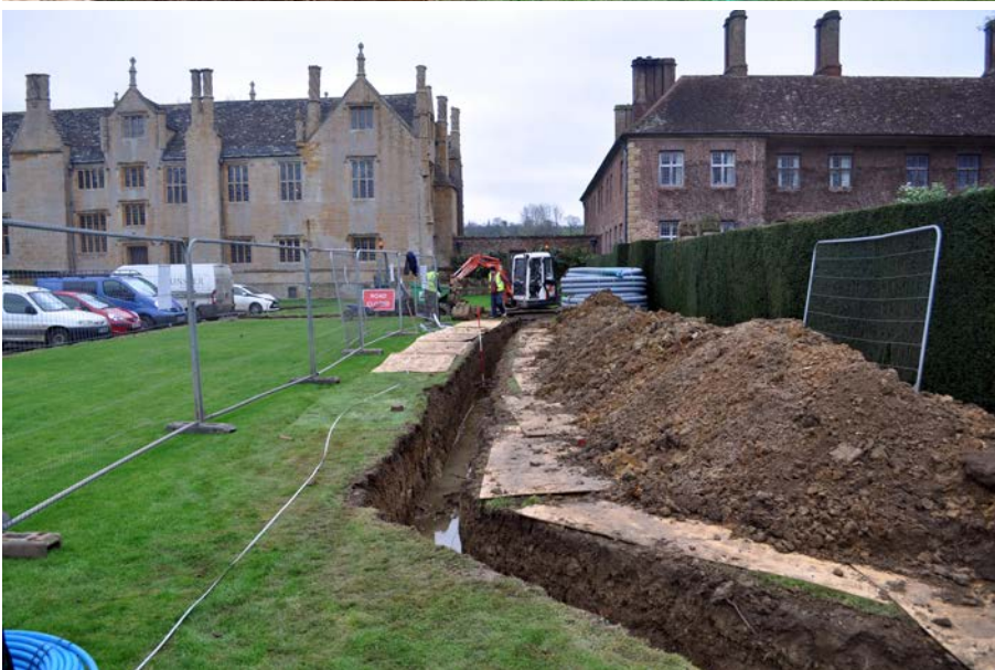
Plate 3: Course of new heat main trench running across north lawn, viewed from NNW. 2m scales.
