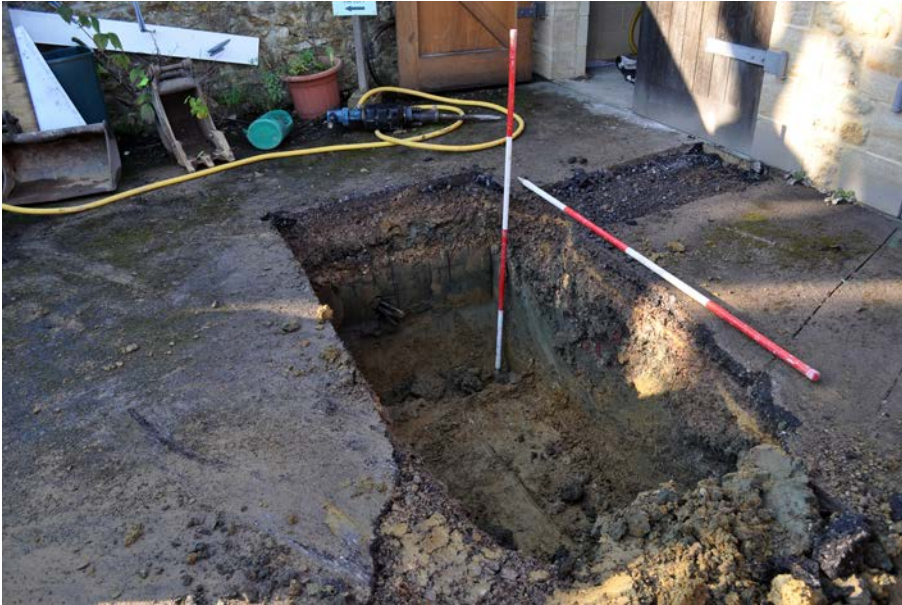
Plate 1: New heat main trench where it enters new boiler room in garages, viewed from E. 2m scales.
