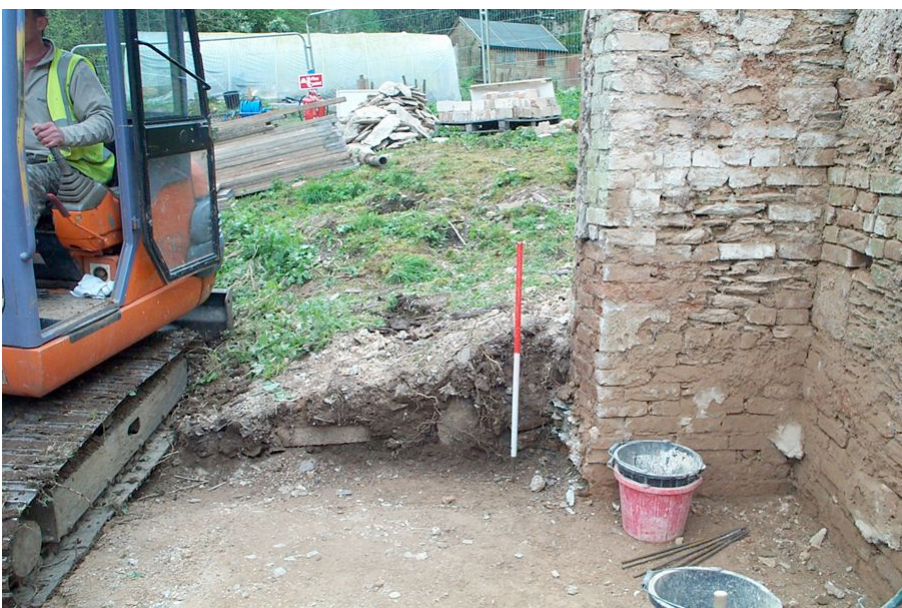
Plate 9: View of material accumulated against the west end of south wall of Room 2.
