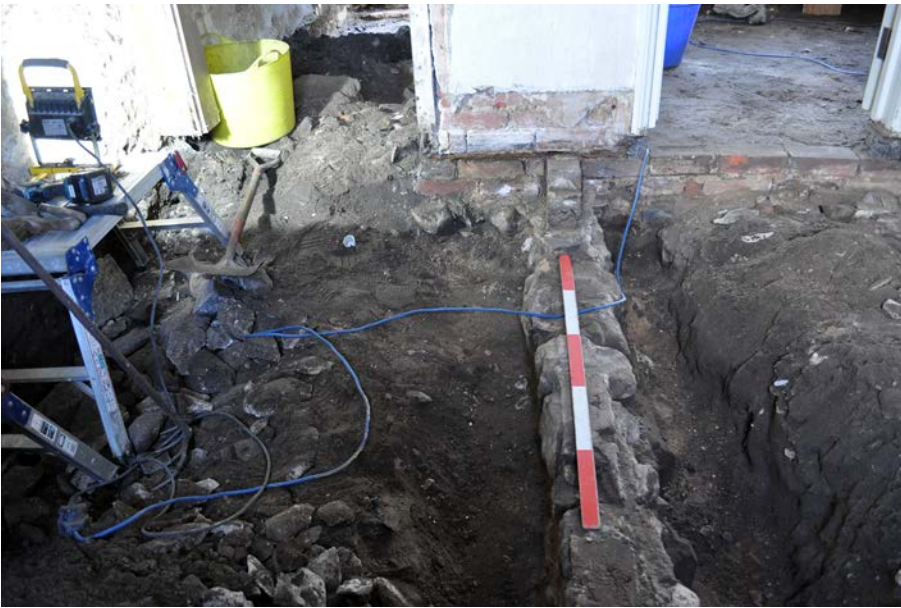
Plate 7: View south along Structure 111 towards internal wall between the north and south rooms. 1m scale.
