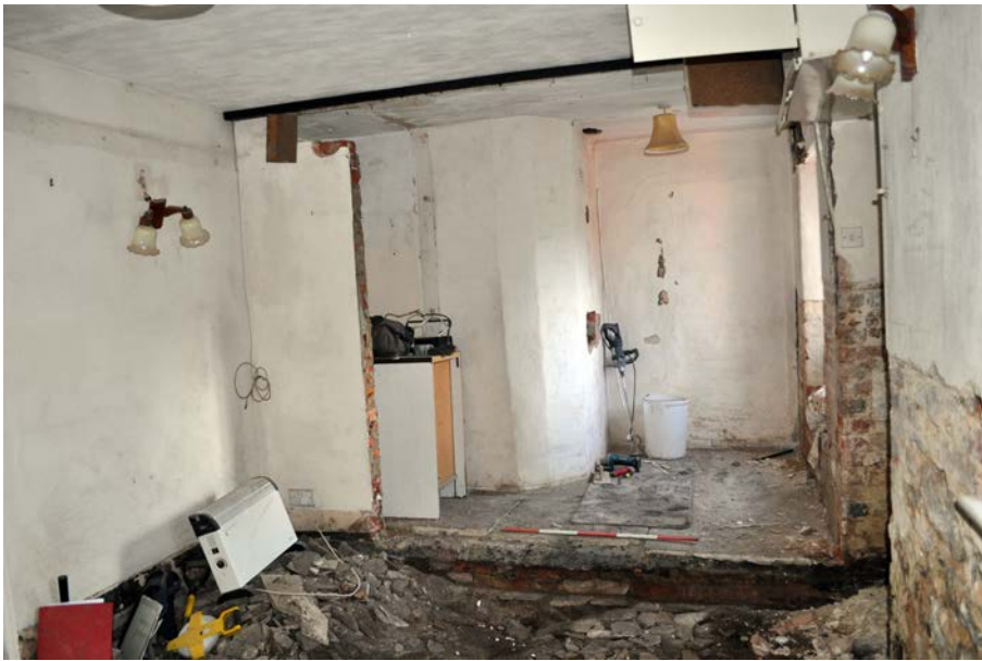
Plate 4: North Room looking west with bread oven and blocked doorway visible in background, together with dwarf wall beneath floor. 1m scale.
