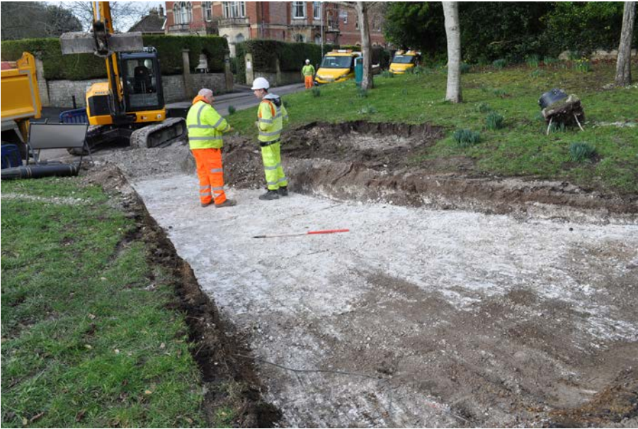
Plate 4: Surface of the natural chalk bedrock 103 in west part of trench. 1m scale.
