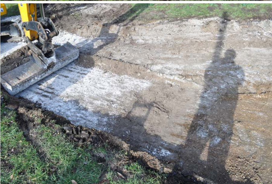
Plate 3: Base of trench during groundworks showing path gravel sub-base 101, over grey silt 102 over natural chalk 103.
