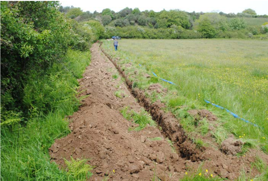
Plate 3: Pipe trench in meadow adjacent to Westhay Farm access track. View from south
