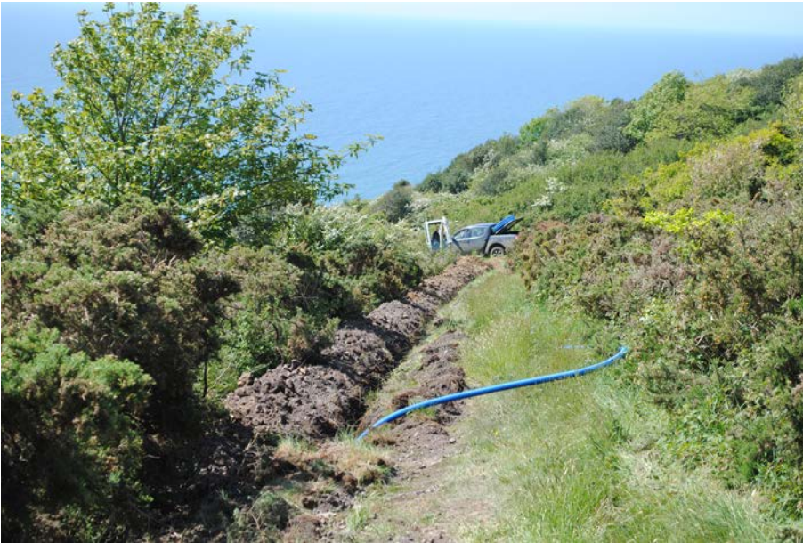
Plate 1: Pipe trench on upper slope of Stonebarrow Hill. View from north east
