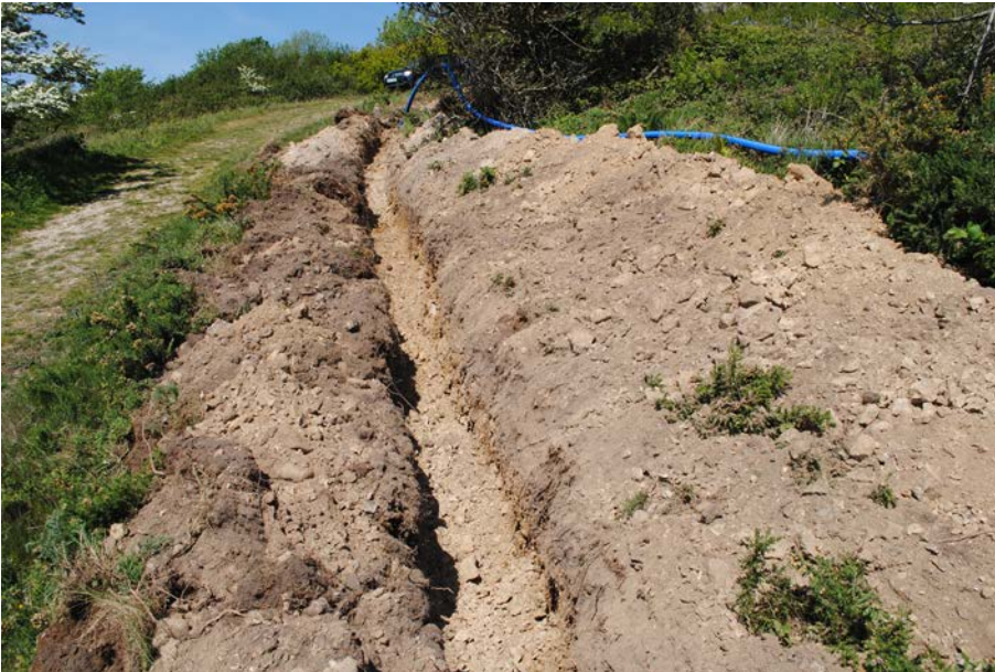
Plate 2: Pipe trench adjacent to trackway on lower slope of Stonebarrow Hill. View from south east
