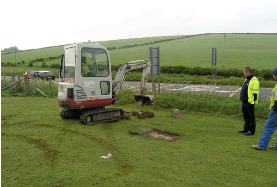
Plate 1: General view of area of pipe burst, viewed from southeast.
