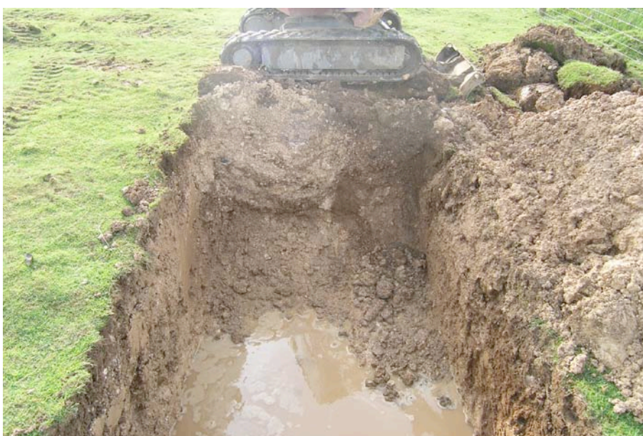
Plate 3: View of trench during excavation, with pipe trench visible to left. View from east.
