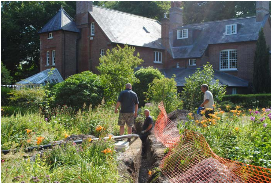
Plate 2: Work on the service trench through the garden north east of Max Gate, looking south west.
