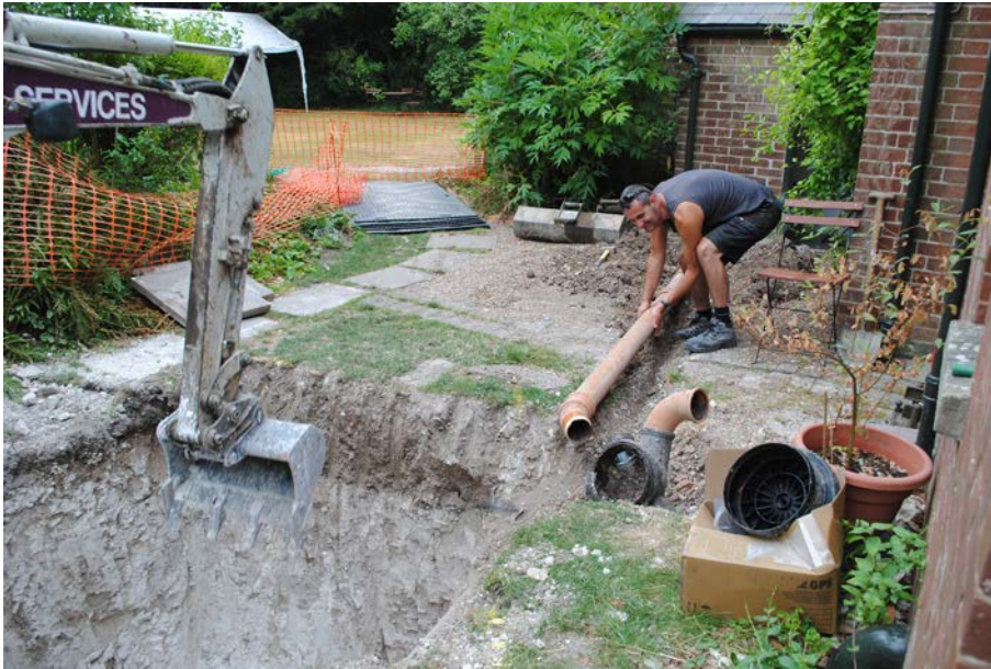
Plate 1: Excavations for the pump chamber adjacent to the east side of Max Gate House looking south.
