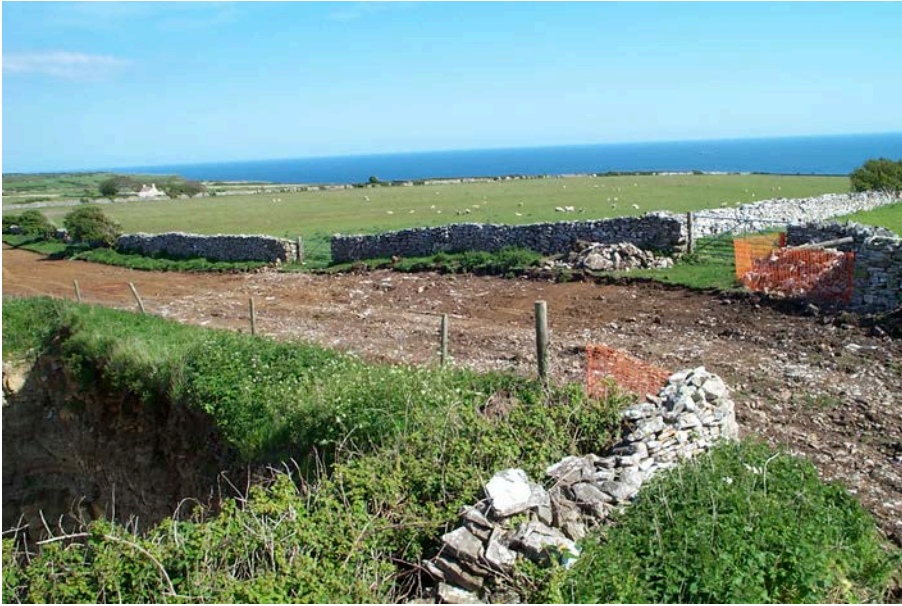
Plate 1: West end of haul road in Blacklands Field showing position of burnt clay feature 11.
