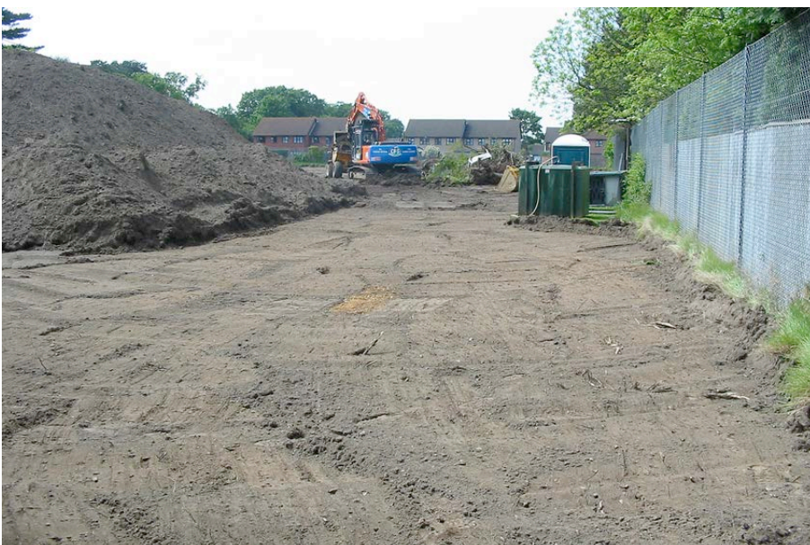
Plate 3: Southern end of site, looking northwest, with the remains of an engineer's testpit in middle foreground.
