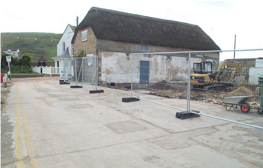
Plate 2: General view of former stable block and northern area of the site, looking east.
