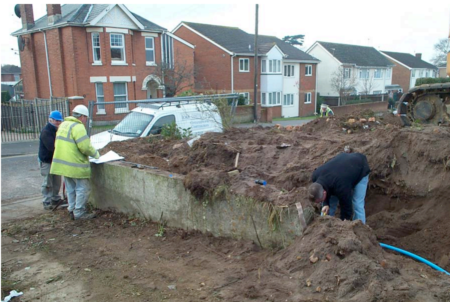
Plate 3: View of deposits at the street frontage during the insertion of a water pipe, looking southwest.
