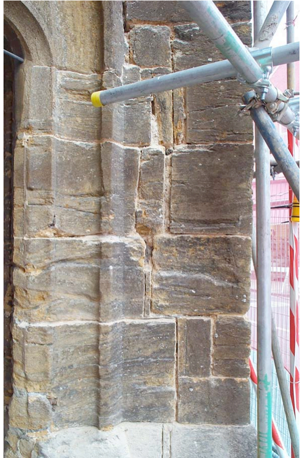
Plate 2: Detail of south face of NE buttress showing differences in mortar.
