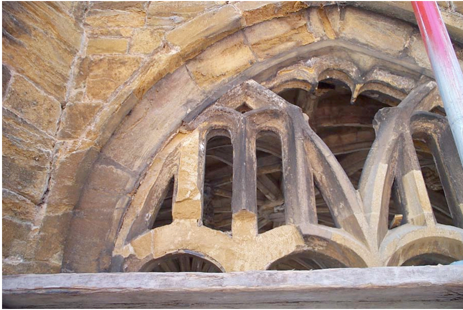
Plate 4: Detail of tracery in NW face during removal of stone, showing remnants of lead came.
