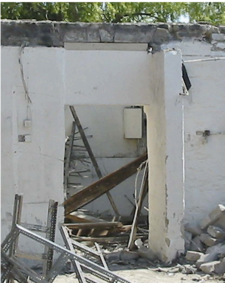
Plate 6: Detail of blocked window and inserted doorway in east end of north elevation.
