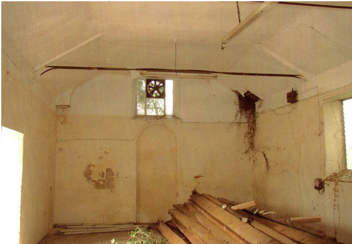
Plate 16: East end of interior prior to removal of ceiling (photo by Betterment Properties (Weymouth) Ltd)
