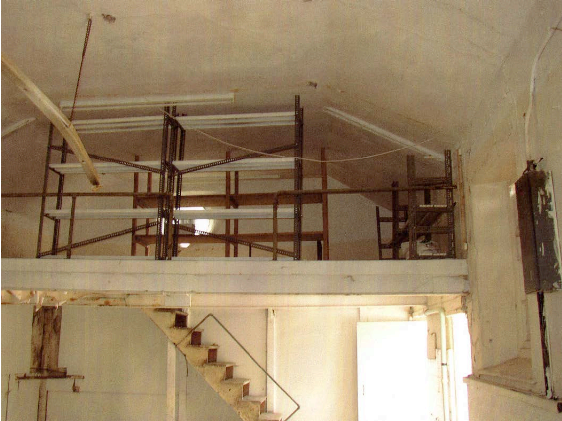
Plate 17: West end of interior and gallery prior to removal of ceilings (photo by Betterment Properties (Weymouth) Ltd)
