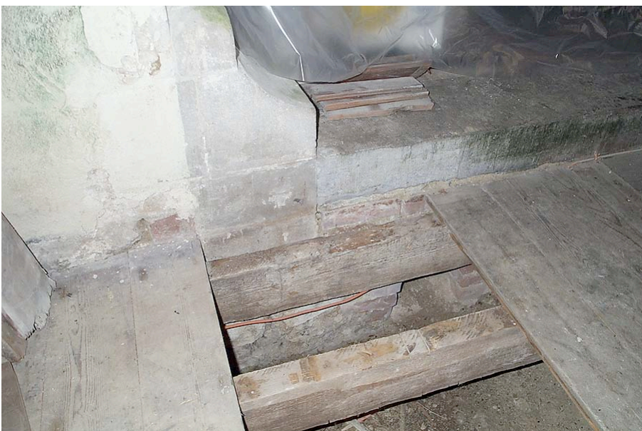
Plate 6: View of 19 th century work below floor in west end of nave, from east.
