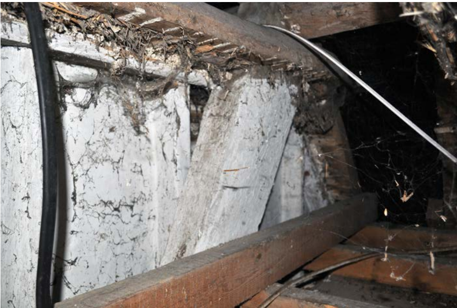
Plate 41: Detail of south end of Truss 1 showing whitewashed strut and partition below removed ceiling level.
