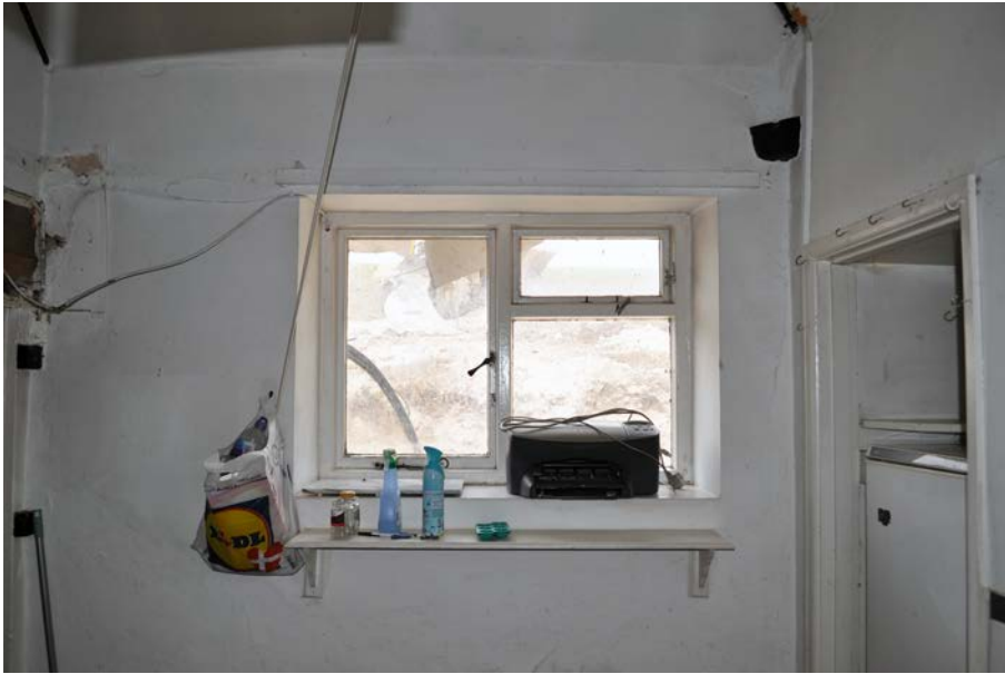
Plate 28: North end of Room 3 with window W8 and larder to right. Note exposed part of dragon tie in corner.
