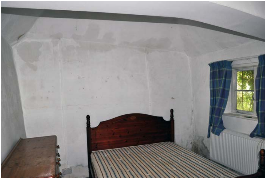
Plate 35: Room 6 looking south with window W4 to right and boxed-in truss above.
