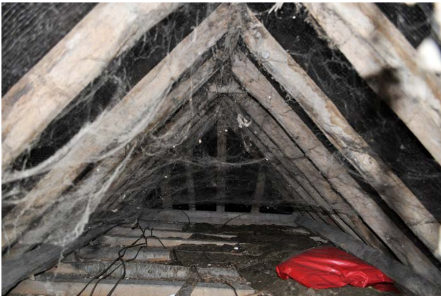
Plate 39: View south along roof space in N-S range with truss 4 in middle distance.
