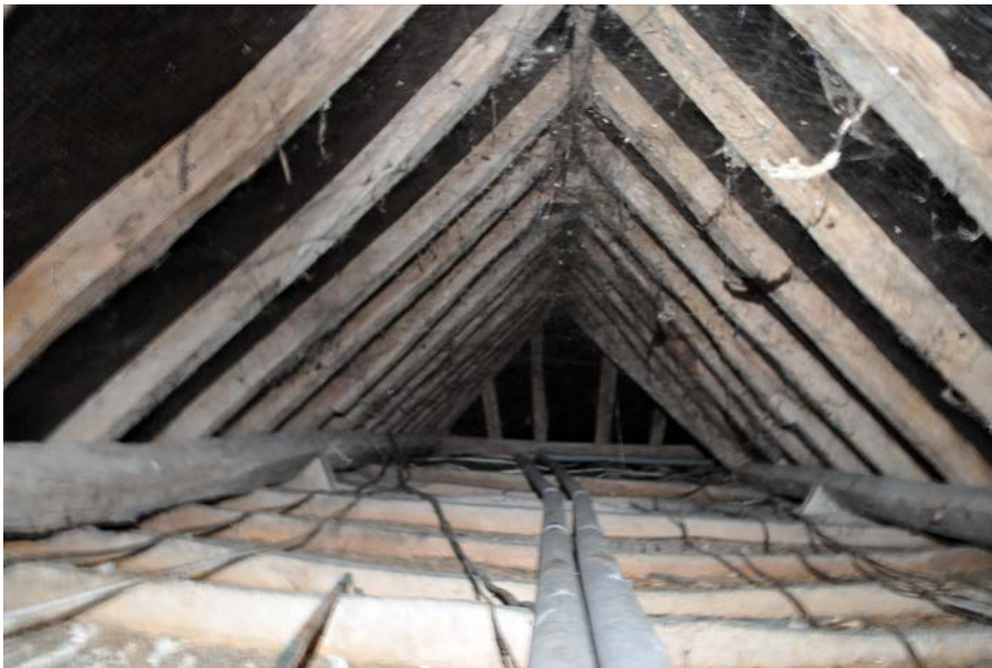
Plate 38: View east along roof space of E-W range showing rafters and Truss 2 (identifiable by ends of struts claspings purlins in middle distance).
