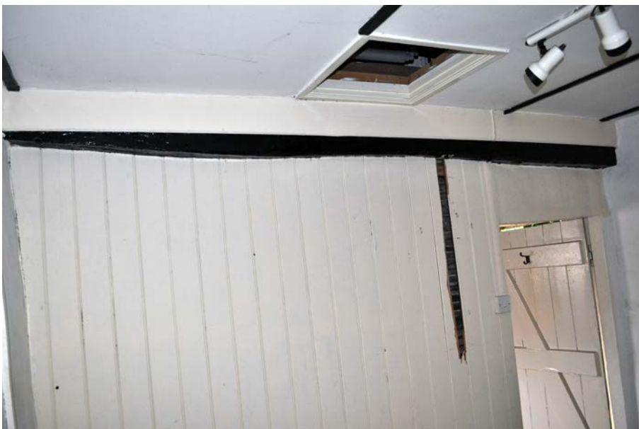
Plate 24: East side of Room 2 showing exposed part of Truss 1 and timber cladding below, with door D2 to right. Note also hatch into roof space in ceiling.
