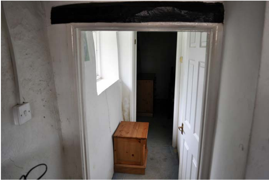
Plate 34: Corridor (Room 5) viewed from Room 3 looking towards Room 6, with window W5 to left.
