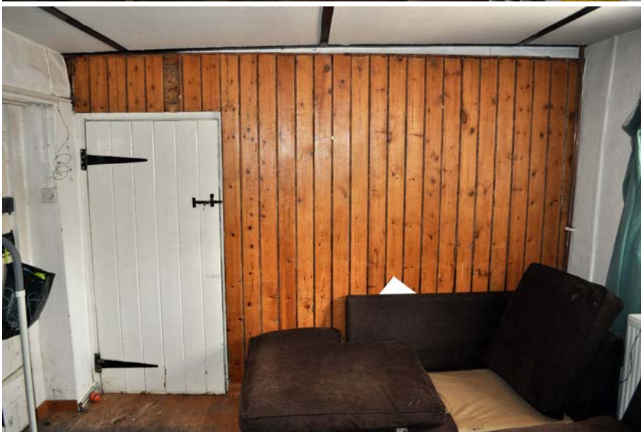
Plate 21: West side of Room 1, showing modern timber cladding, with door D2 to left.
