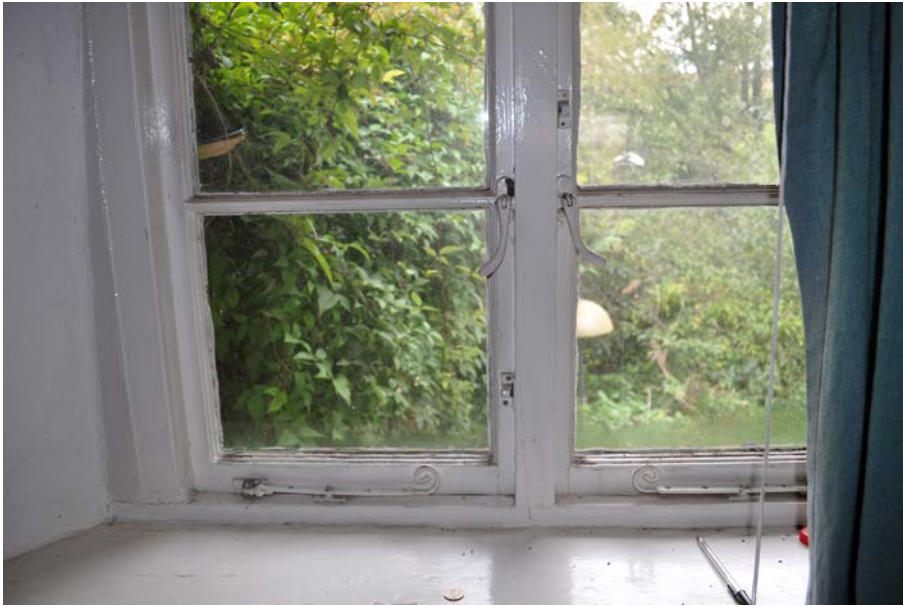
Plate 22: Detail of Window W2 showing window furniture.
