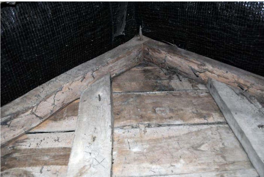
Plate 42: Upper part of west face of Truss 1 and timber partition above former ceiling level.
