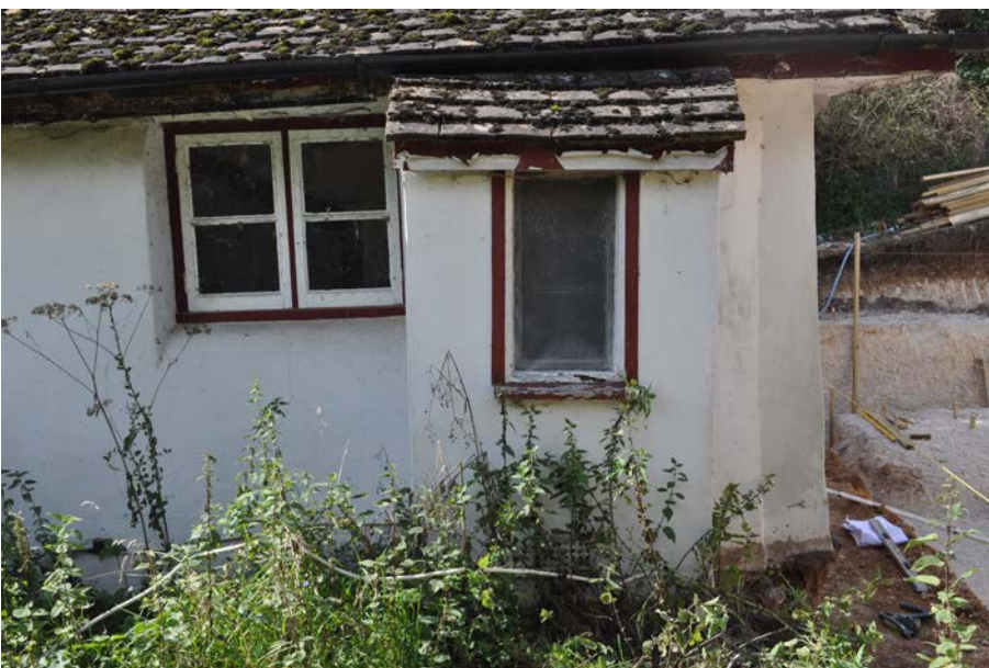
Plate 8: Inserted larder at north end of east elevation. Window W6 to left.
