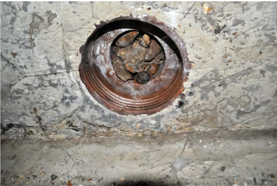
Plate 20: Detail of blocked vent in roof of air raid shelter.
