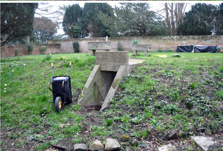
Plate 15: North entrance to air raid shelter, built into side of former castle ditch, looking SE.
