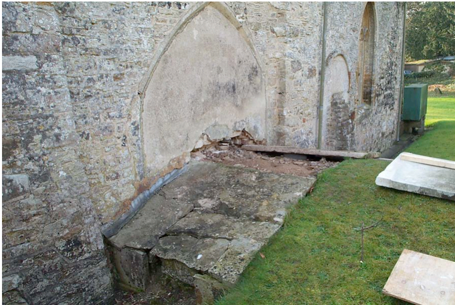
Plate 1: View of stone structure of the Lambert Tomb during stone removal. Viewed from northeast.
