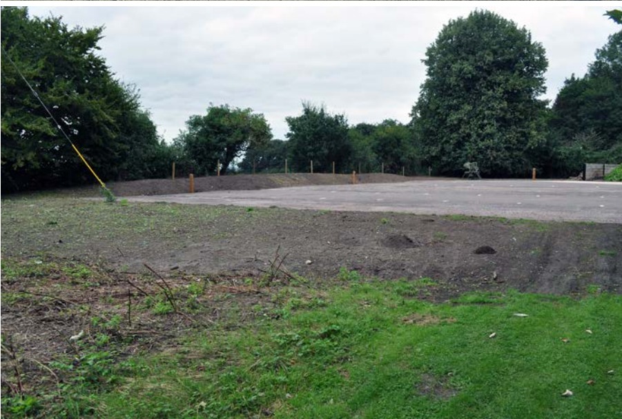
Plate 9: New Staff Car Park, looking north east, showing build up in levels.
