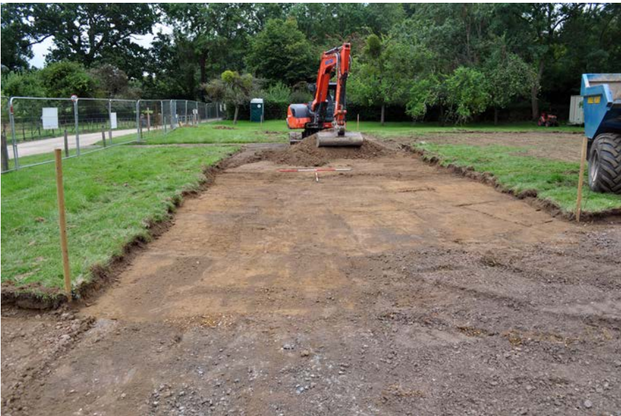
Plate 5: View of topsoil stripping in Orchard overflow car park, looking south. 2m scales.
