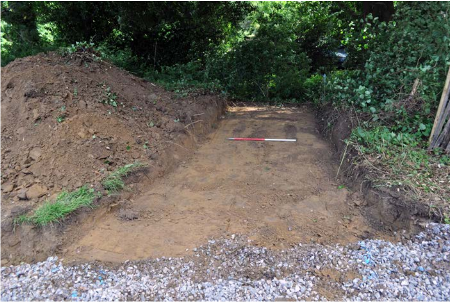
Plate 4: View of area of reduced ground for the installation of the new pedestrian bridge in Helens Close. 1m scale.
