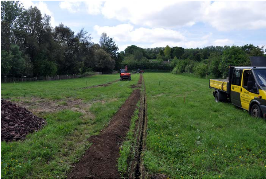
Plate 1: General view of electricity trenches for new car park in Helens Close, looking south.
