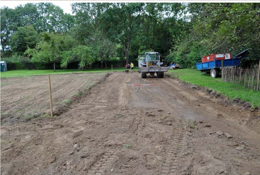
Plate 6: View of topsoil stripping in Orchard overflow car park, looking south. 2m scales.
