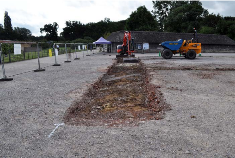
Plate 7: Beagles Car Park during initial stripping, looking south, with possible earlier road just in front of machine bucket.
