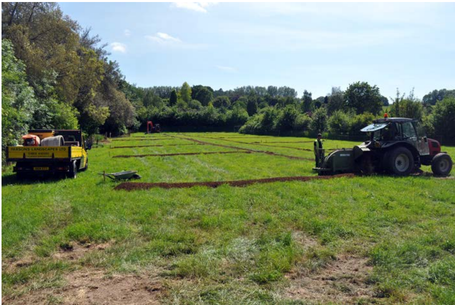
Plate 2: General view of electricity trenches for new car park in Helens Close, looking south.
